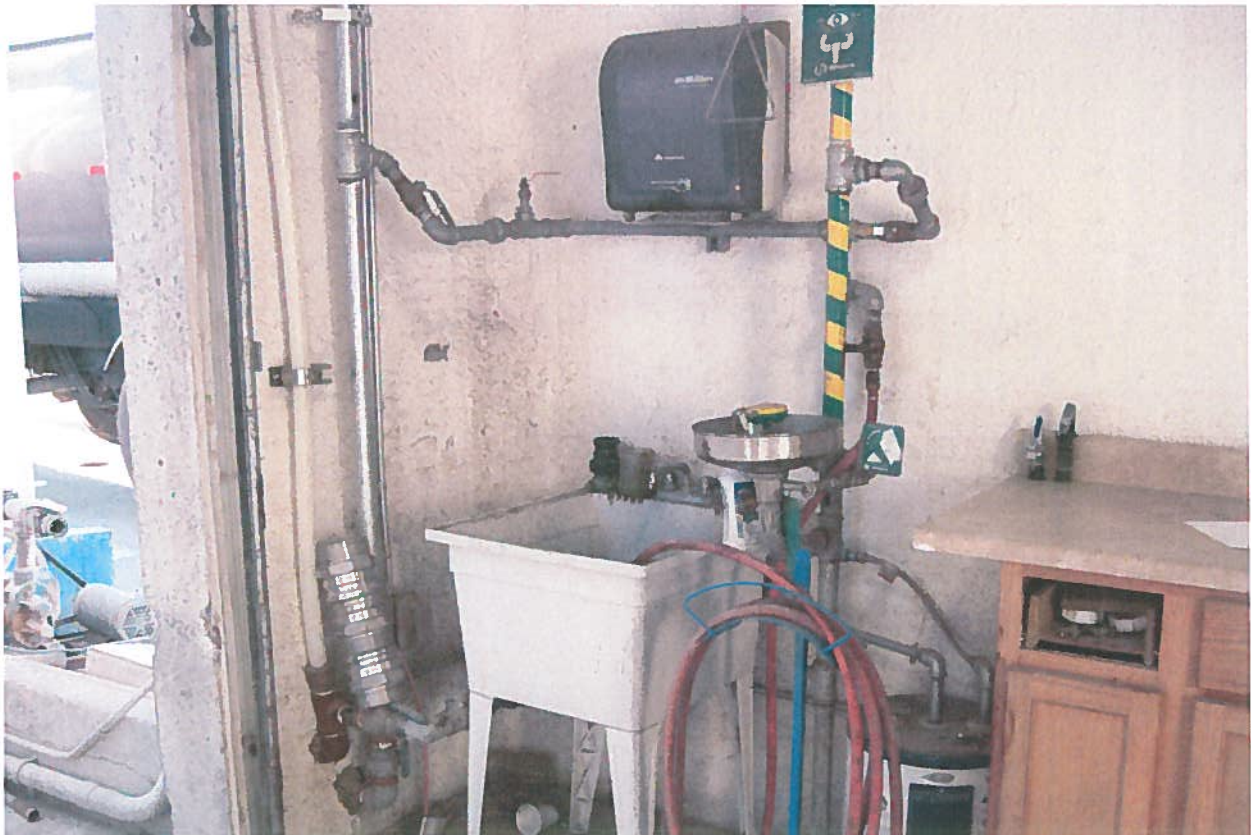
Below: Emergency eye wash, sink and small hot water heater
