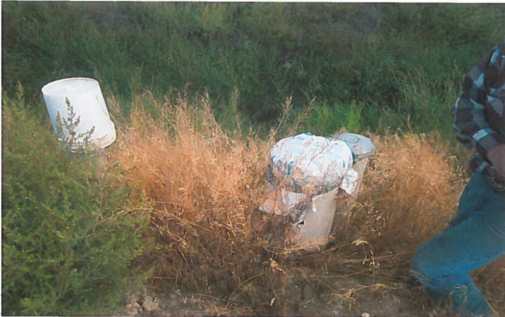
Pump and motor is about 20 feet deep in this casing [middle of photo] , adjacent to Sage Creek.
