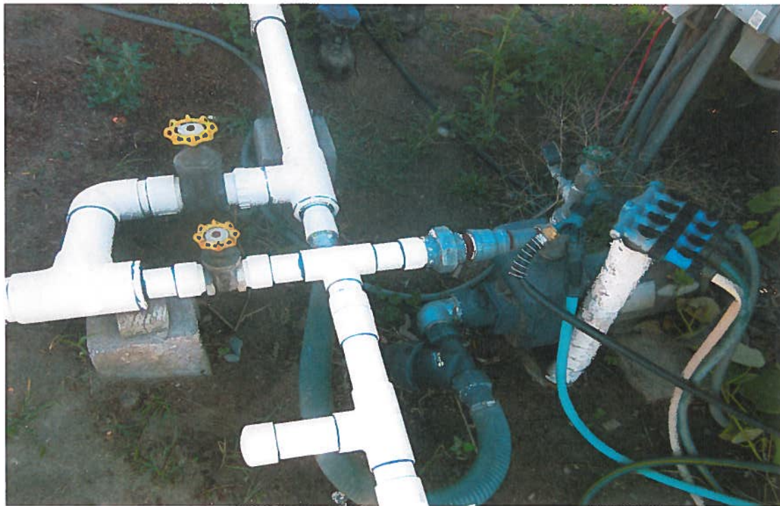
Three hp pump and irrigation piping for irrigation of Mr. Sherman's property.
