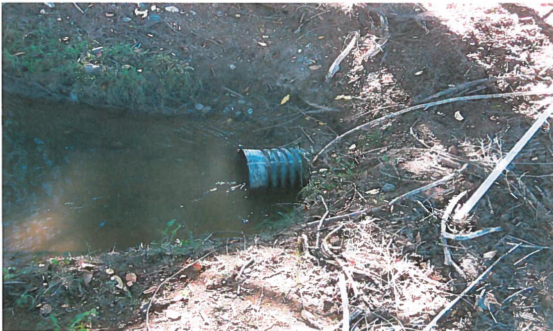
Buried pipe from the Ruby Drain to the "drop" at the POD.
