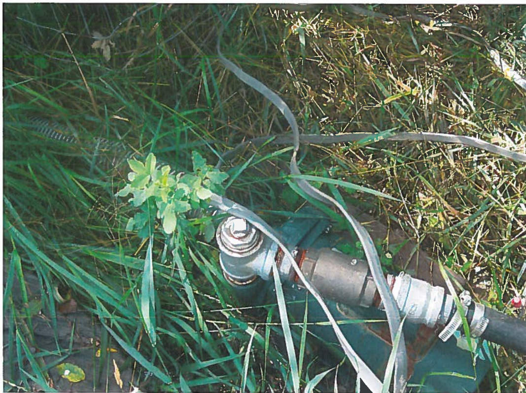
Pump and motor. Pipe from cistern/POD seen left.
