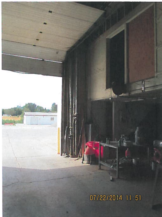
Flowmeter on vertical pipe at right of door.
