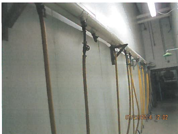
Hoses for plant wash down
