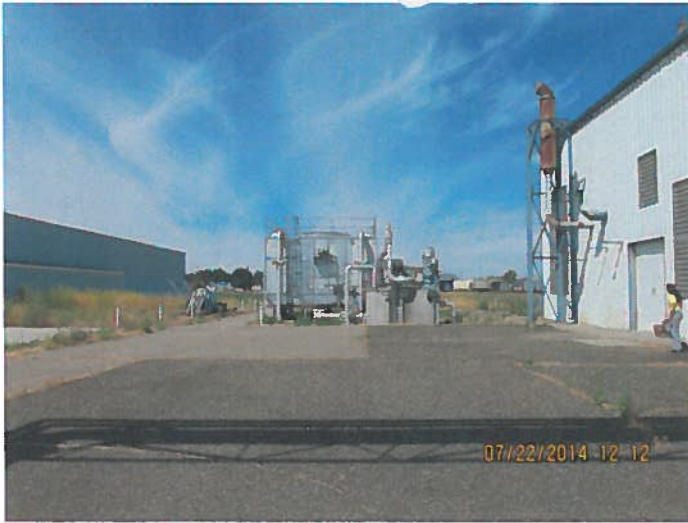
Cooling tower south of co-generation plant
