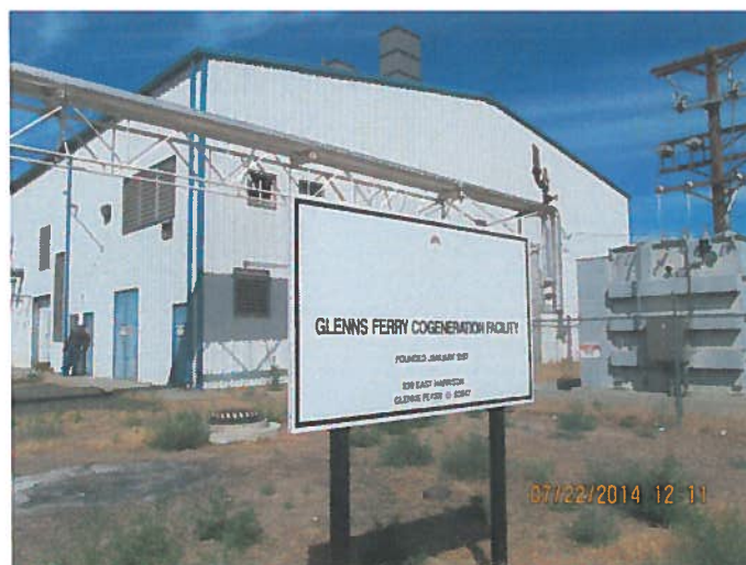
Gas-fired Co-Generation plant. Three overhead pipes carry water from storage tank, steam to processing plant and steam condensate to co-generation plant.
