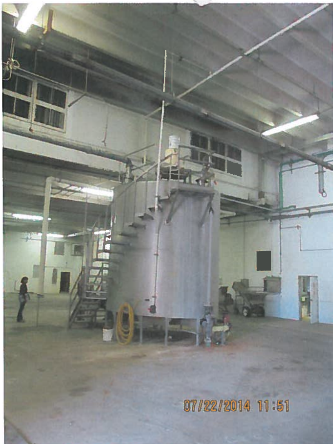
Water storage tank inside plant
