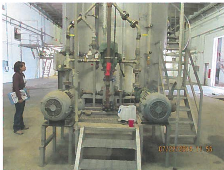
Two 40 hp pumps (L & R) for plant use. 15 hp pump (center) to co-generation plant
