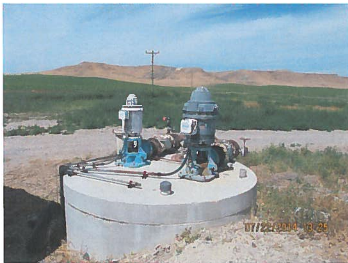
Pumps from storage pond
