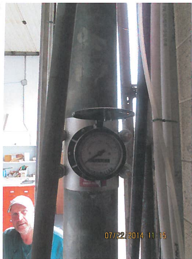
Flowmeter inside south side of plant
