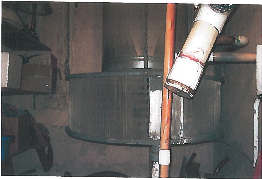
Heat exchange unit in North Building
