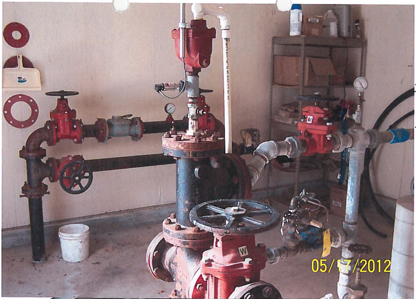
Inside pump house #1
