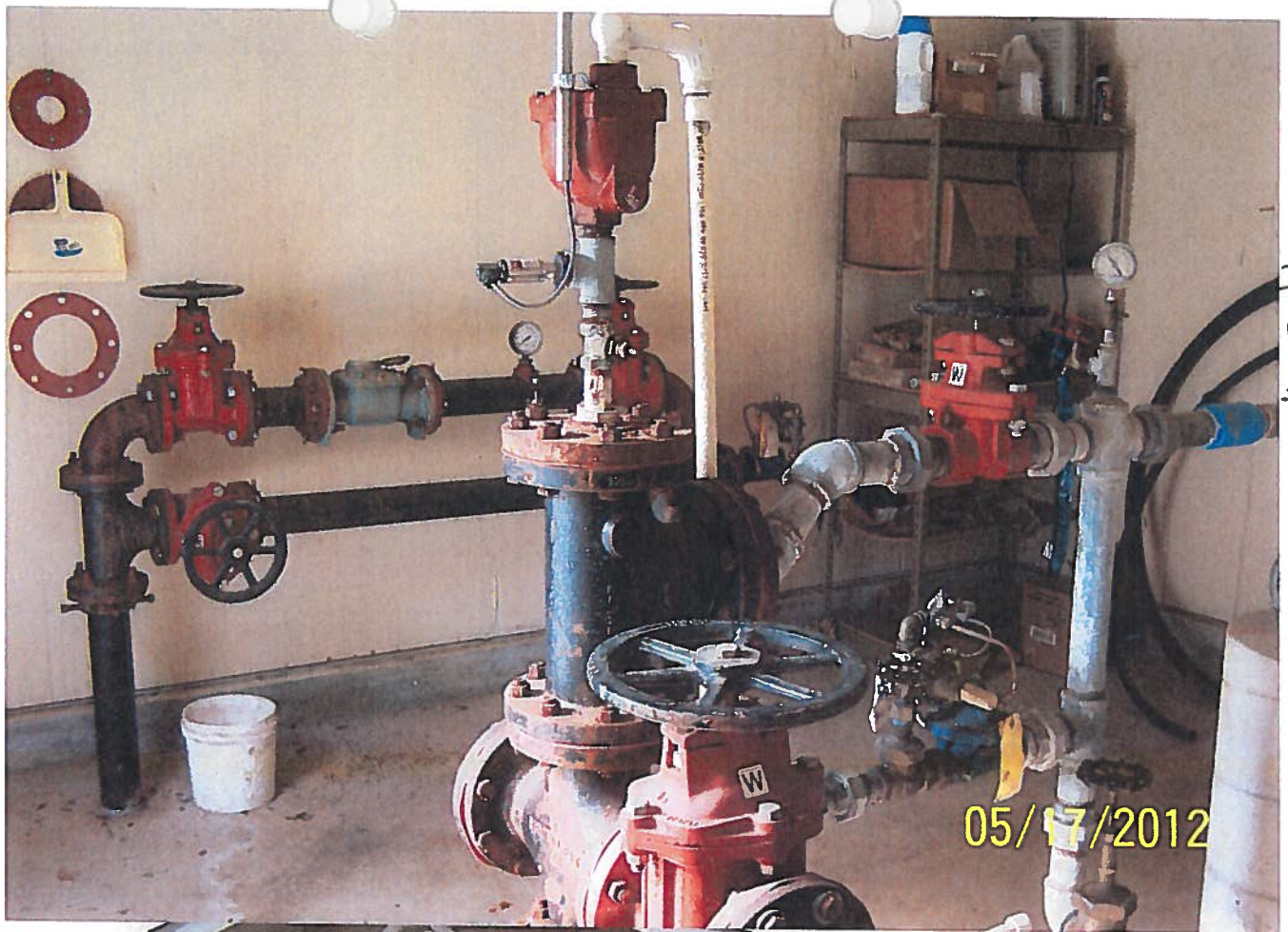
Inside pump house #1
