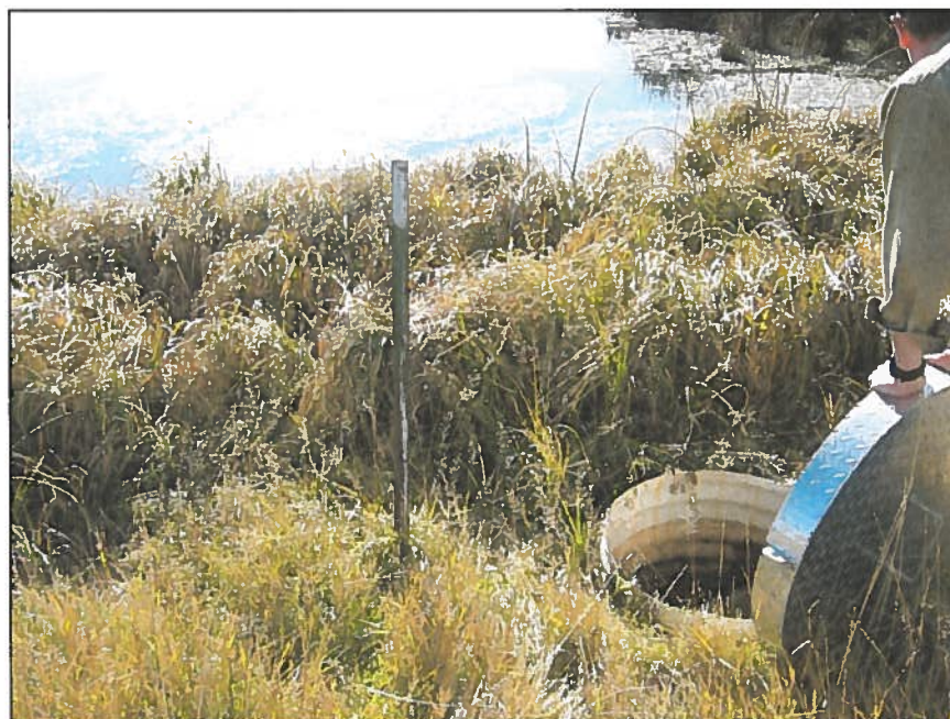
Figure 10: Foster Pond outlet control. Overflow discharges to Outlet Pond.
