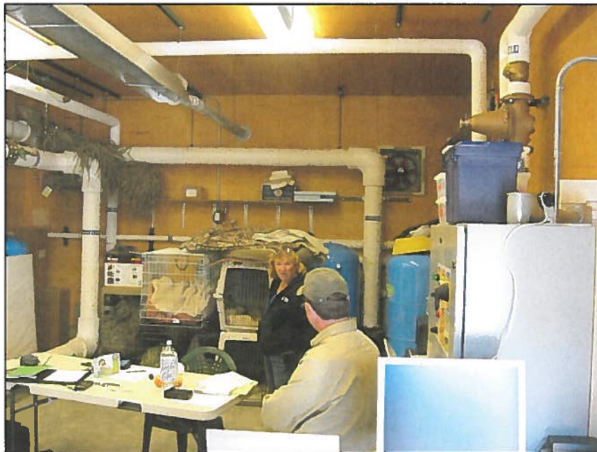
Figure 4: Pump control panel on right.
