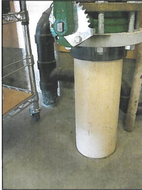
Figure 3: SPF ultrasonic flowmeter was installed on this pipe.
