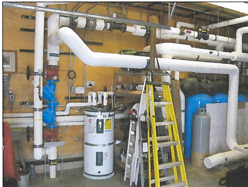
Figure 2: Plumbing in well house.
