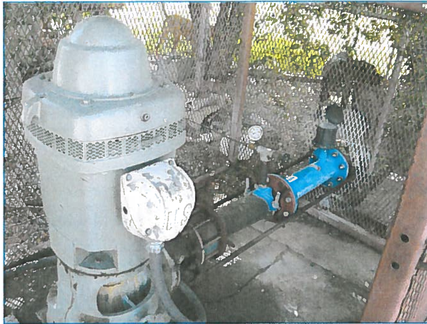
Figure 7: 30-hp turbine pump and plumbing.
