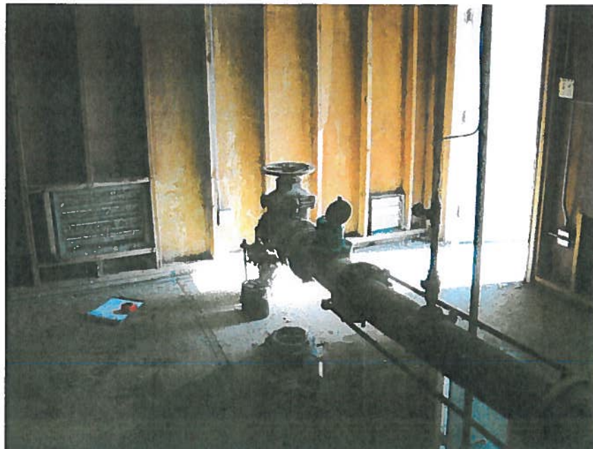
Figure 20: Plumbing and flowmeter.
