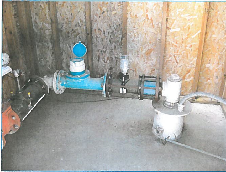
Figure 11: 20-hp submersible pump and plumbing.
