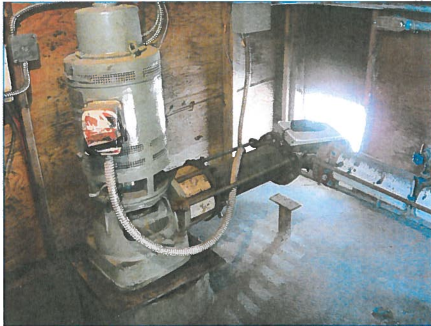
Figure 13: 20-hp turbine pump and plumbing.
