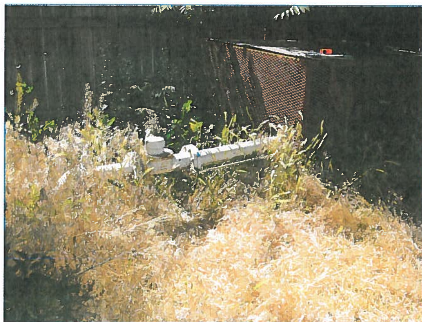
Figure 24: Plumbing and flowmeter.
