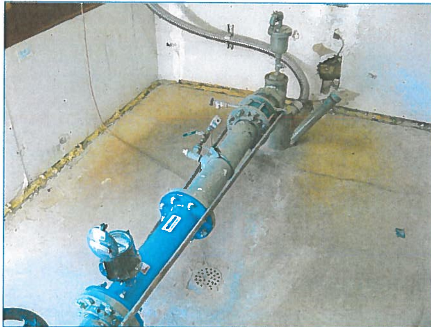
Figure 26: Plumbing and flowmeter.
