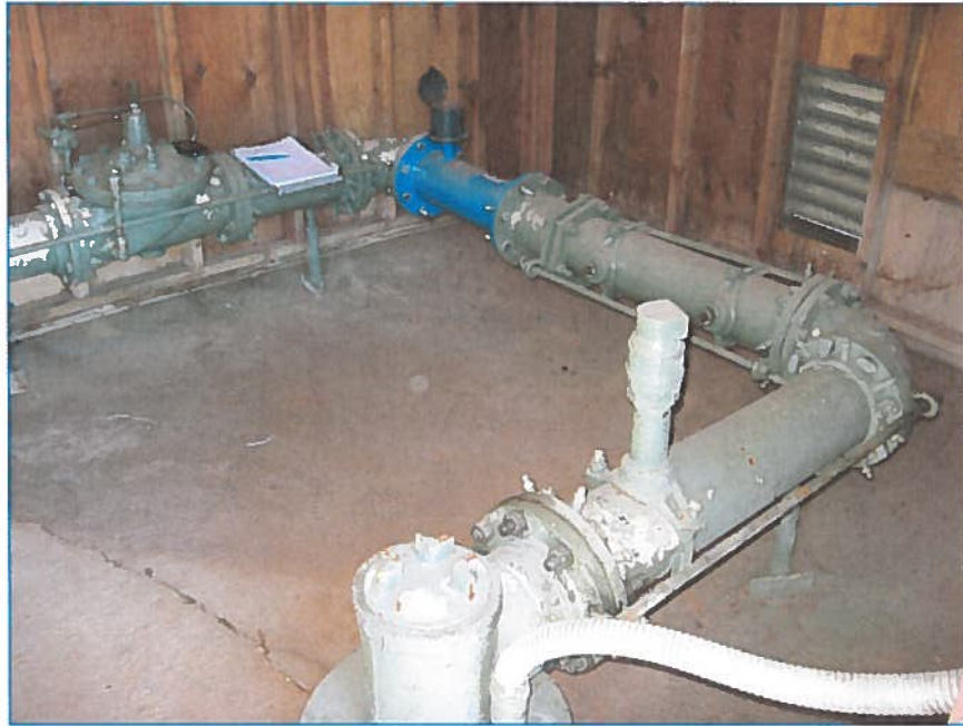
Figure 1: 25-hp submersible pump and plumbing.
