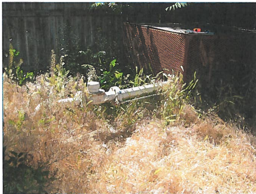
Figure 24: Plumbing and flowmeter.
