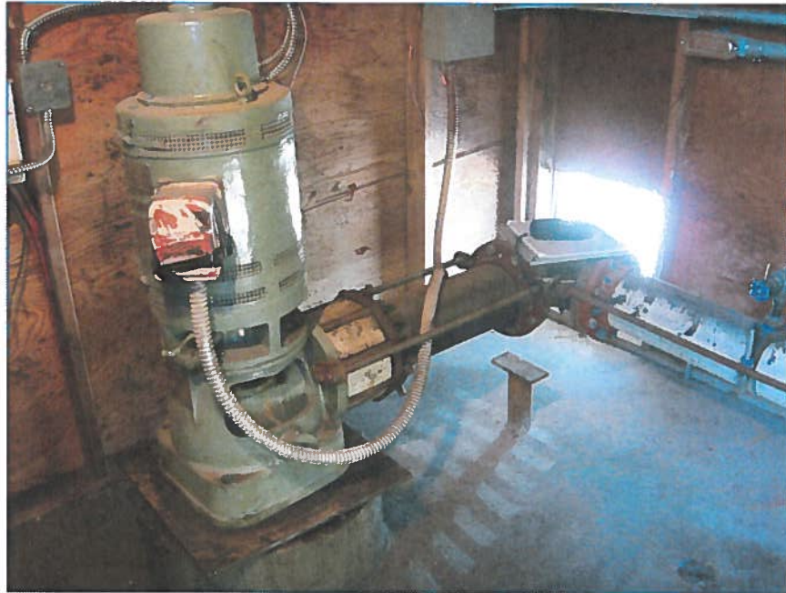
Figure 13: 20-hp turbine pump and plumbing.
