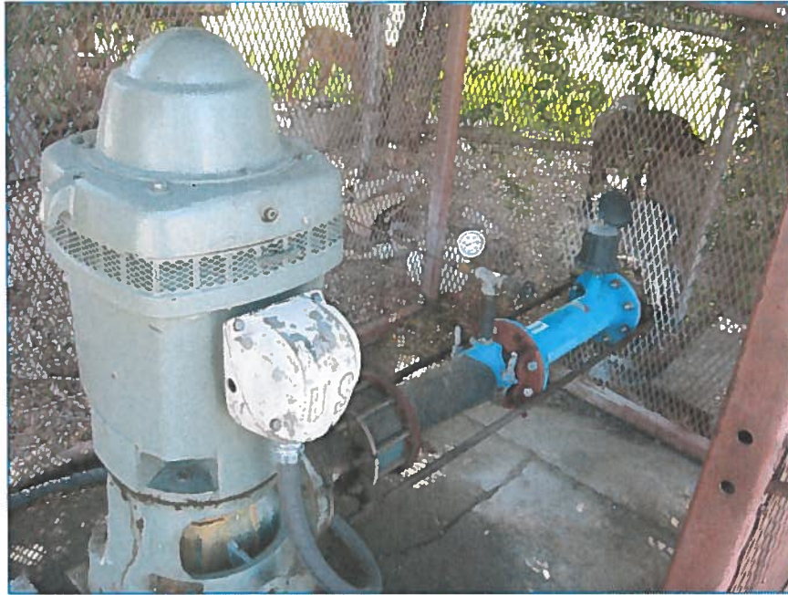
Figure 7: 30-hp turbine pump and plumbing.
