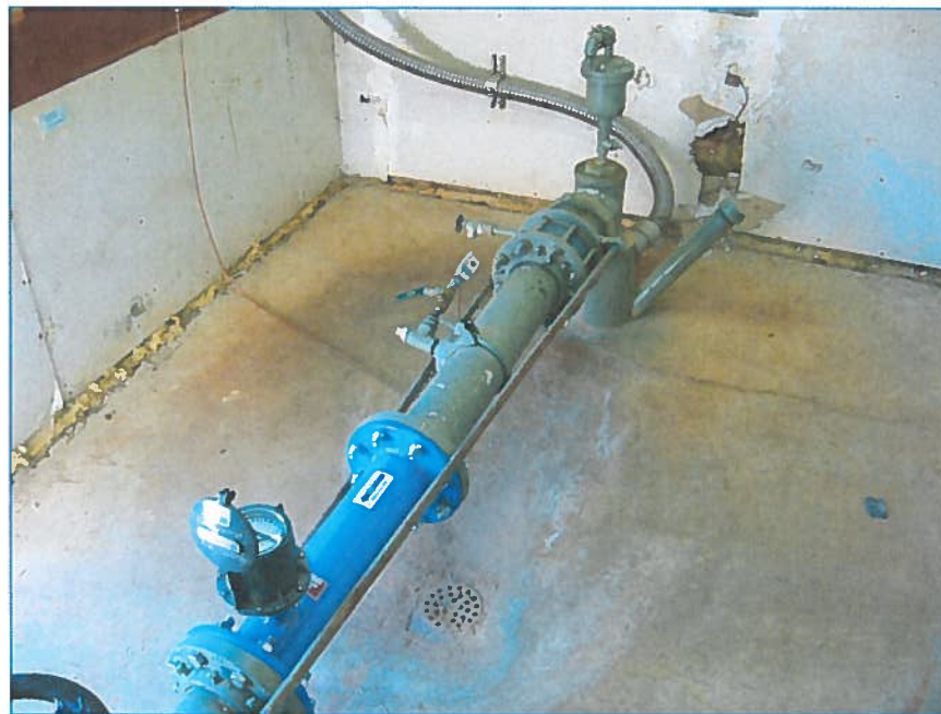
Figure 26: Plumbing and flowmeter.
