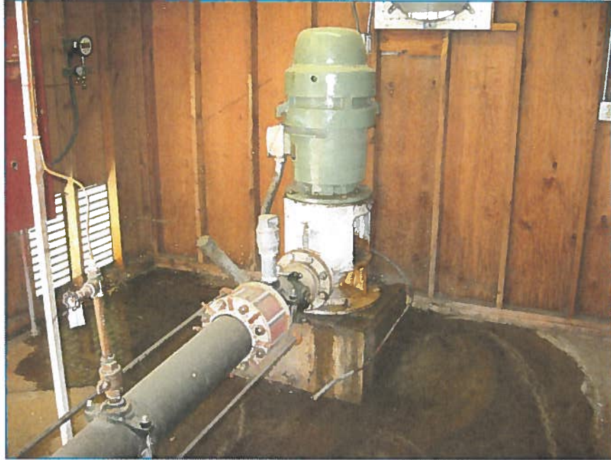
Figure 19: 40-hp vertical pump and plumbing.
