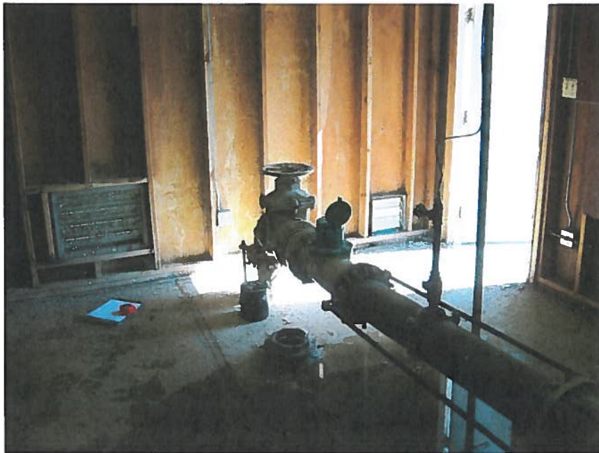
Figure 20: Plumbing and flowmeter.
