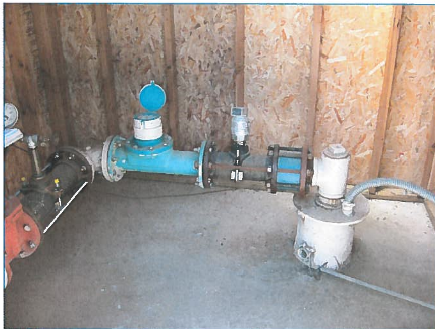
Figure 11: 20-hp submersible pump and plumbing.
