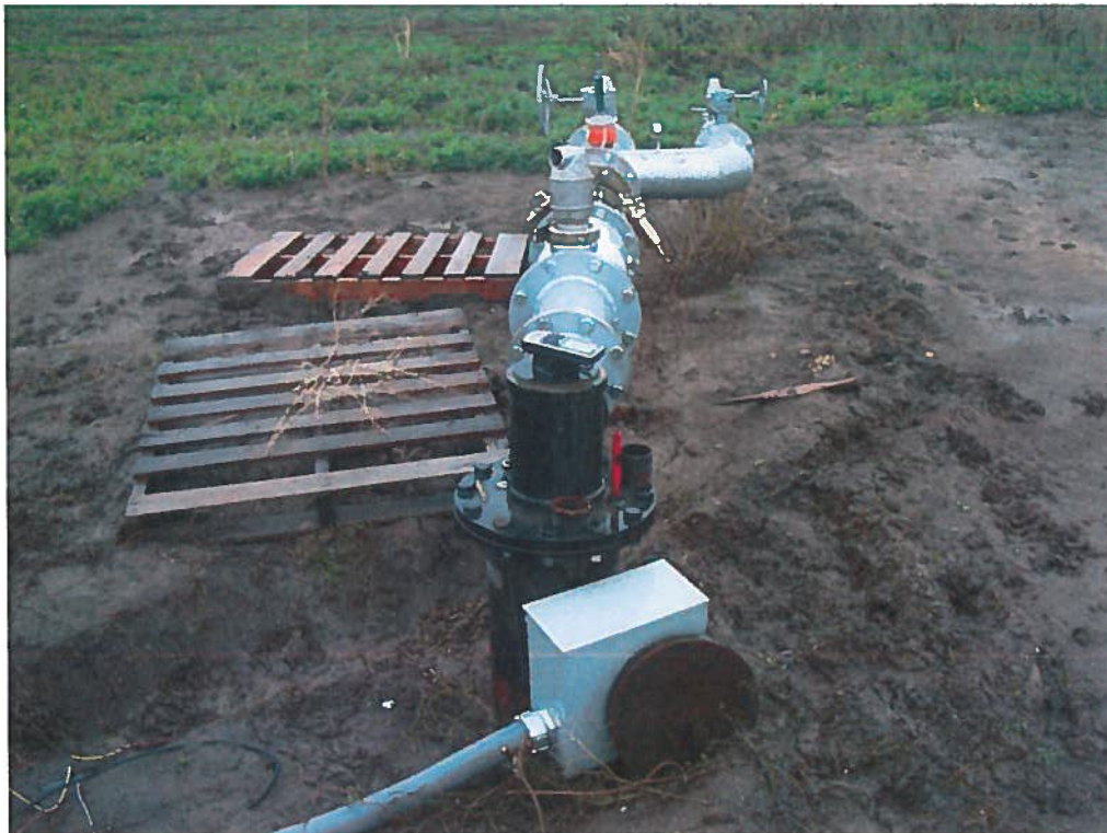
67-15088 Field Exam 10/24/2014: POD well with measurement port (small red tube) facing west. 10 inch line to pivot center valve with 6 inch line off to right.
