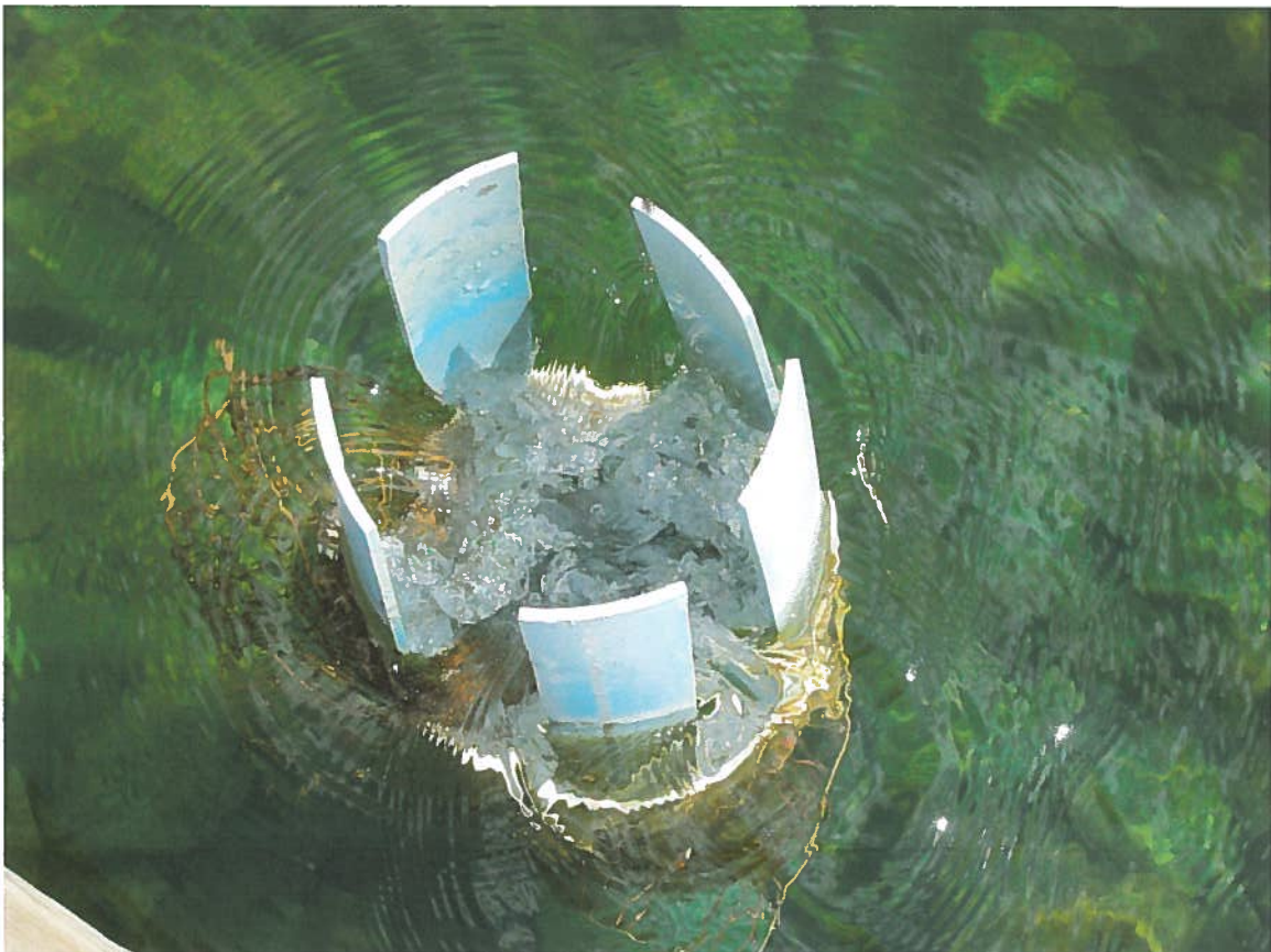
Picture 6: Close up picture of the return flow stand pipe.
