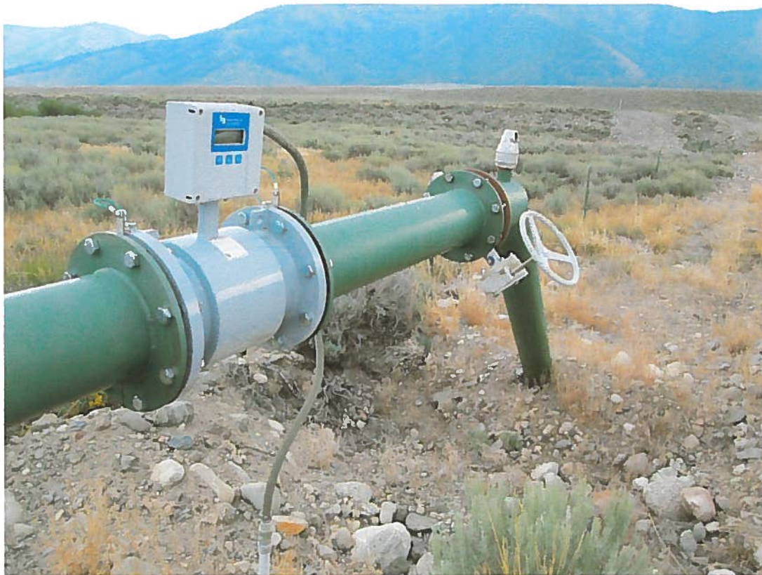
Picture 2: Badger M2000 flow meter installed on delivery pipe to ponds.
