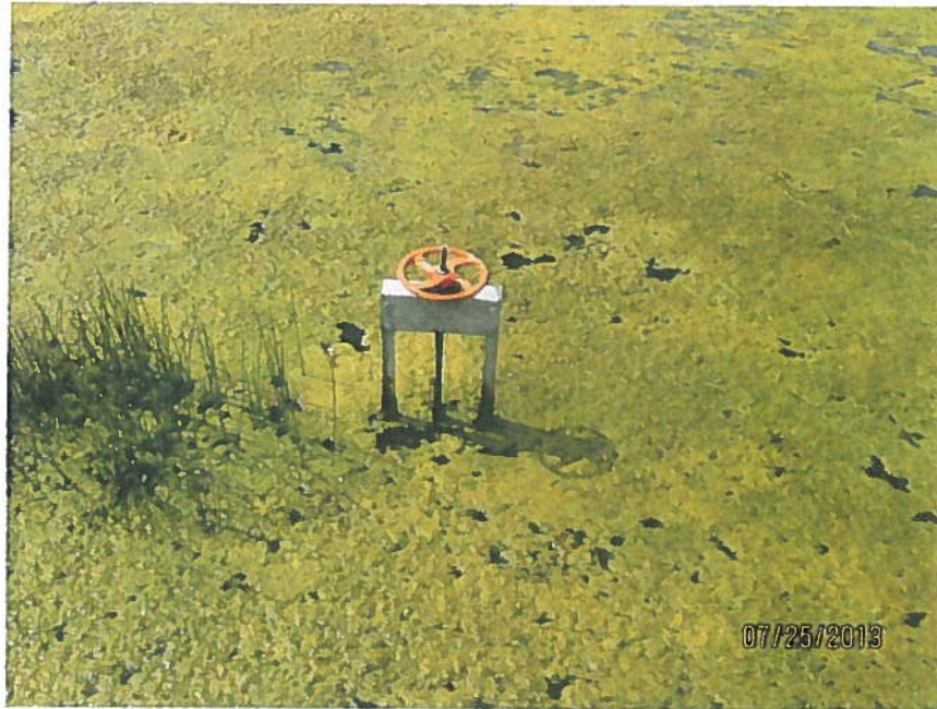
Figure 3: Pond outlet gate valve.
