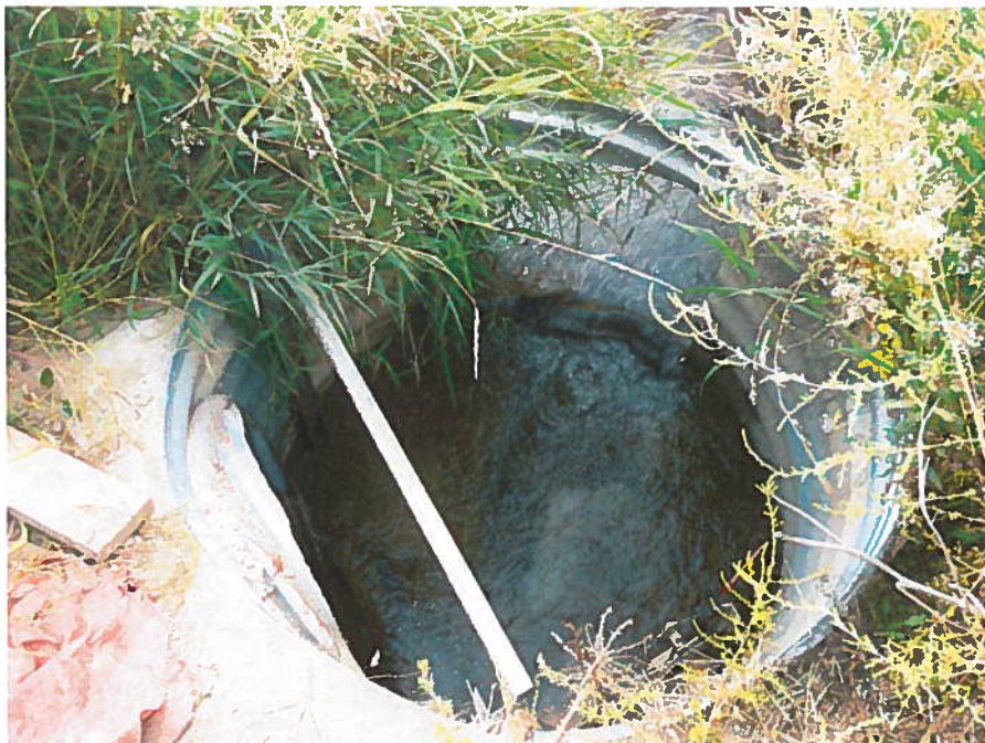
Collection culvert for surface water used on the place of use
