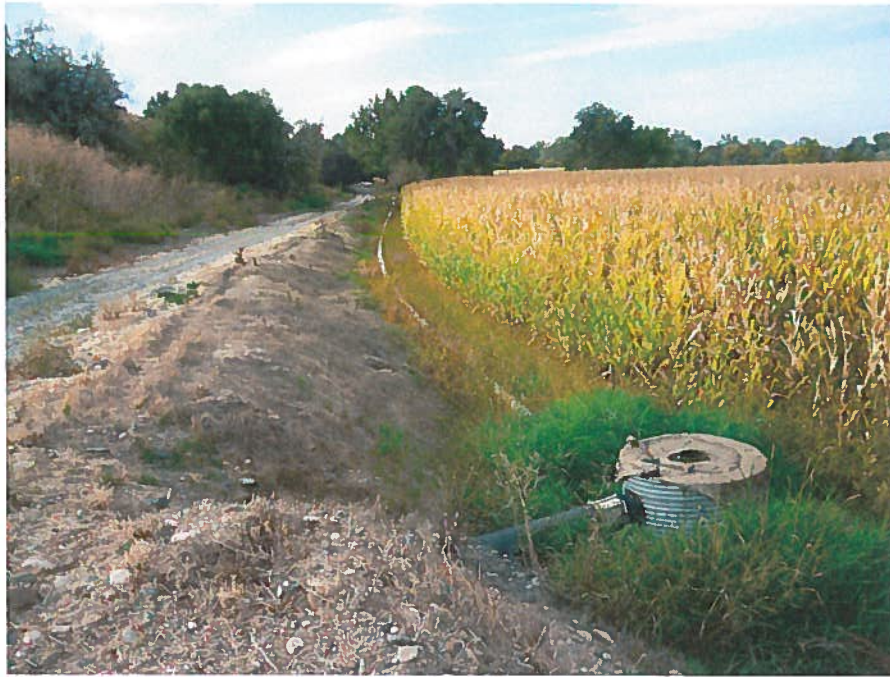
Distribution pipe for surface water bordering place of use
