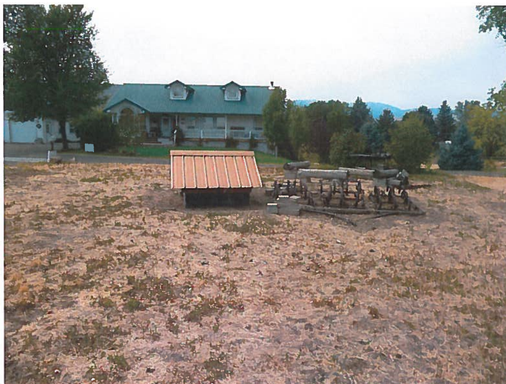
67-14474 Site Visit 9/23/2014: POD well inside small well house with brown roof. House and portion of lawn irrigated in background facing east.
