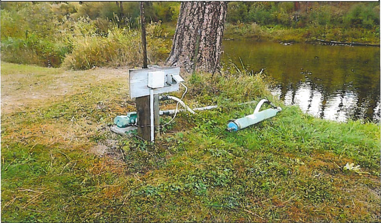
View easterly of the 2-hp centrifugal pump, pressure filter, and power source at the northeast corner of the right holder's parcel.
