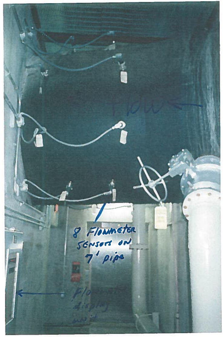
Mainline in power plant with Accusonic flowmeters attached.
