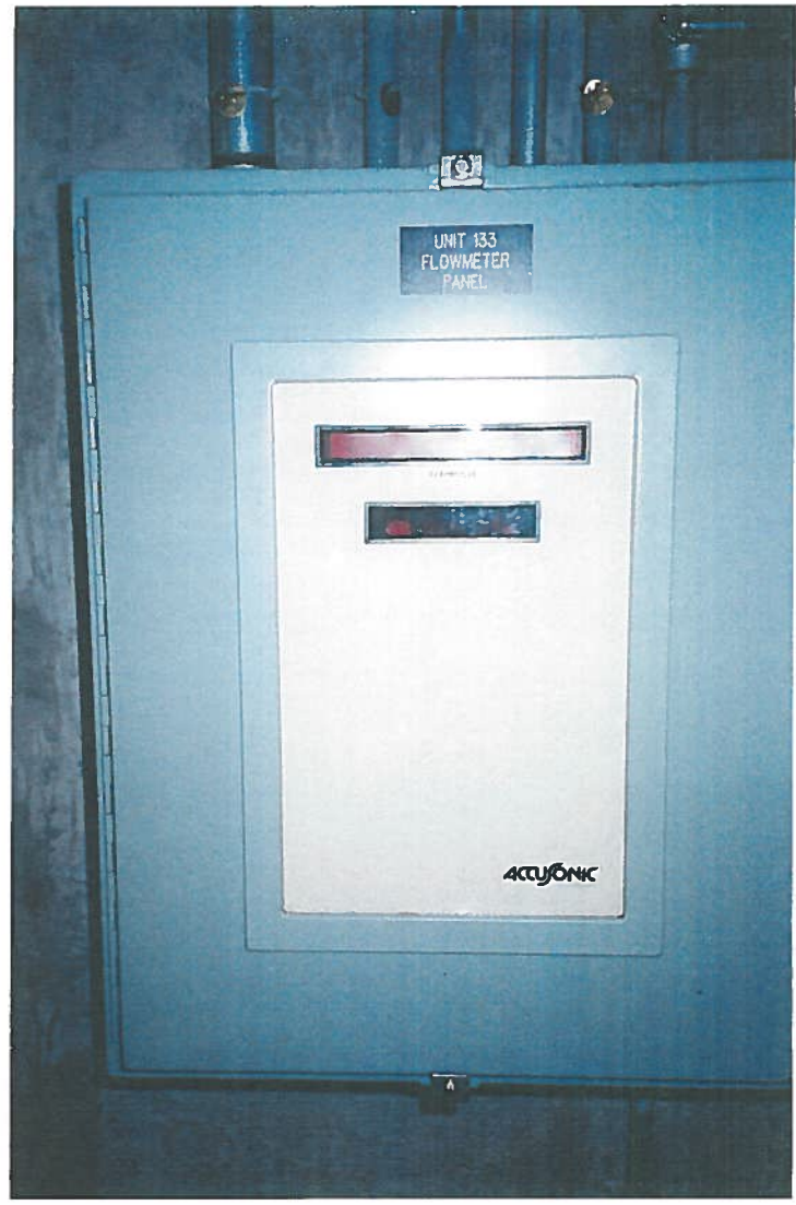
Flowmeter display panel (also at bottom left of photo #3).
