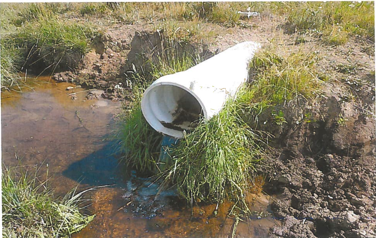
View of the 15" PVC wildlife storage pond outlet pipe. Water is discharged to a drainage/irrigation ditch.
