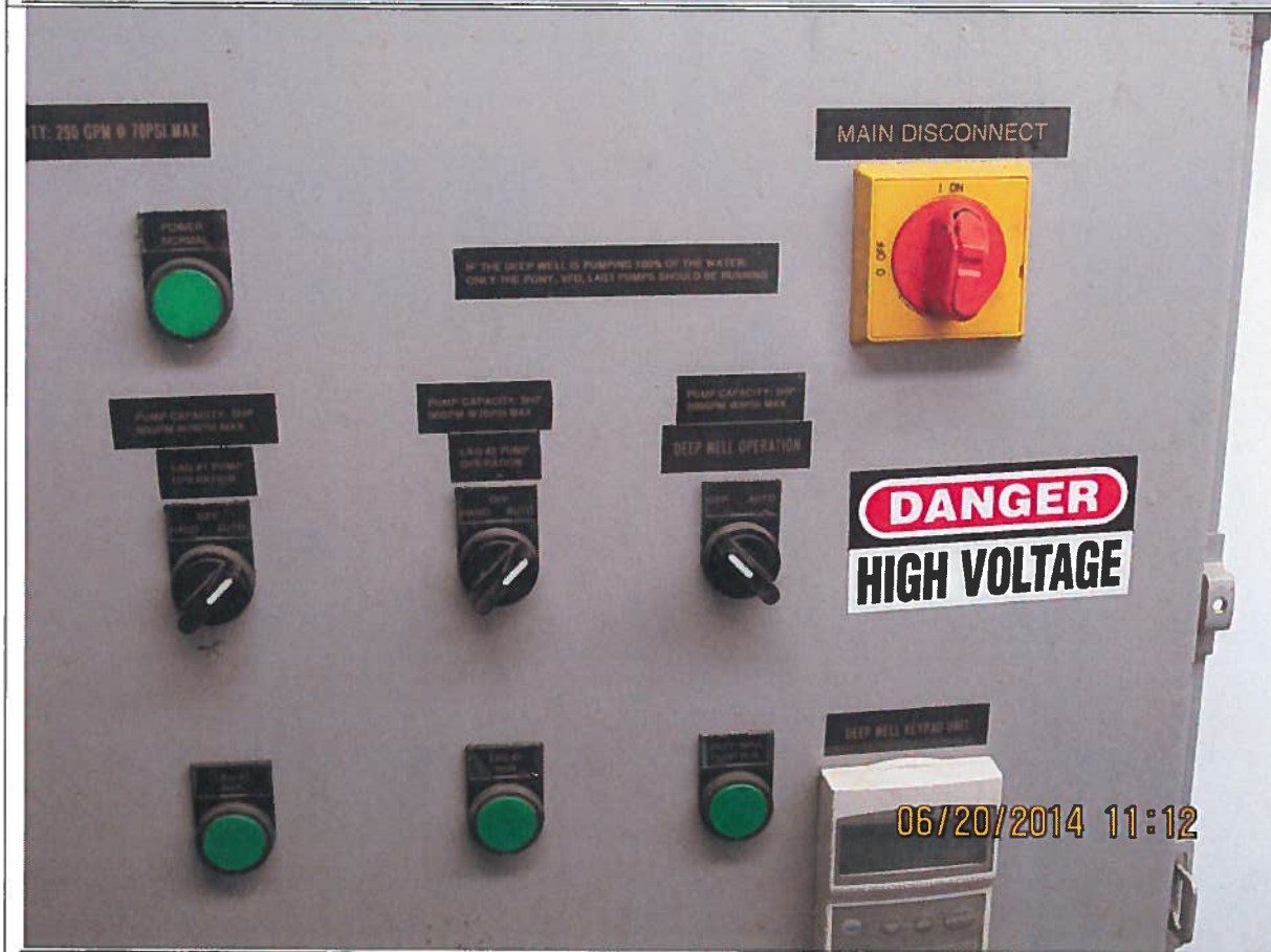
Control panel (right side)
