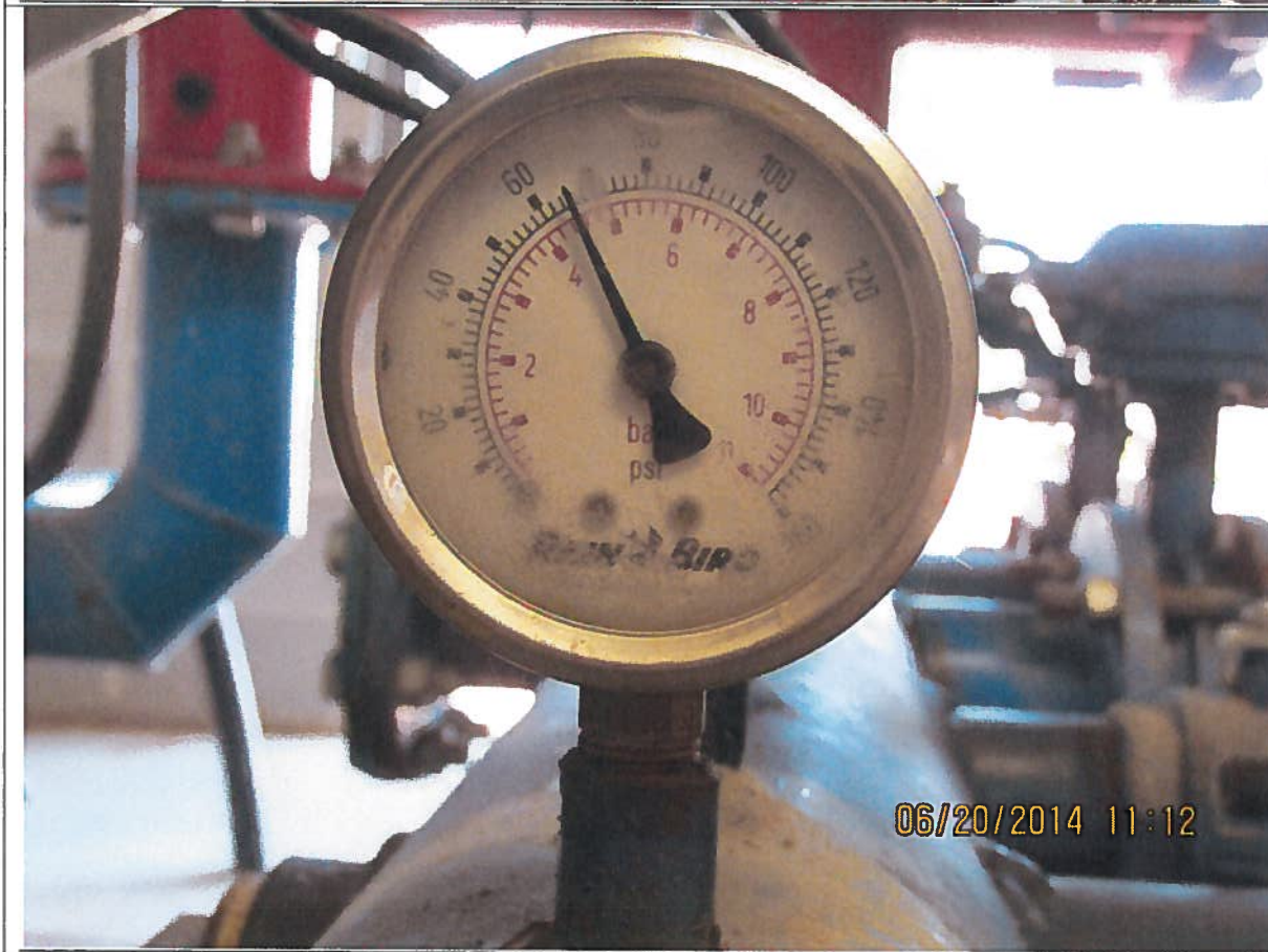
Pressure gauge on system at 65 psi.
