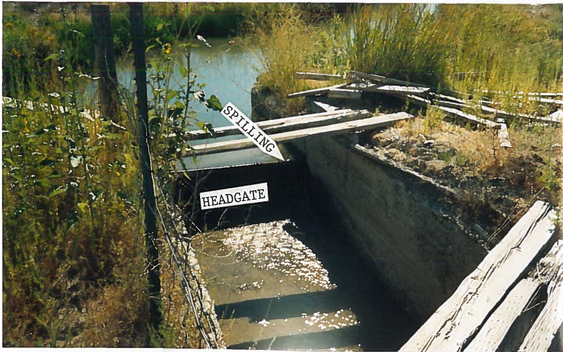
PHOTO ONE- Taken looking east at a headgate used for the diversion of excess water from the Buckaroo Canal into a ditch. There was a small spilling of water through and over the planks installed in the headgate as shown in the photo.
