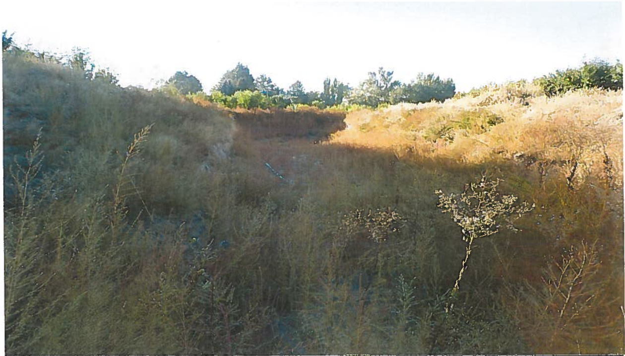
Photo 4 – View southerly from the north end of the storage pond of the thick weed growth on the banks and walls of the storage pond and the upstream slope of the dam.
