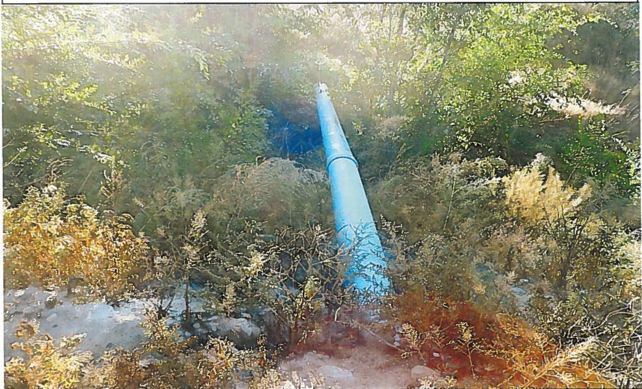
Photo 5 – View southeasterly of the east 12" PVC overflow pipe. The overflow pipe is cantilevered approximately 36' from the top of the downstream slope to the downstream toe near the Escott Drain. No pipe supports were installed to support the overflow pipe sections.
