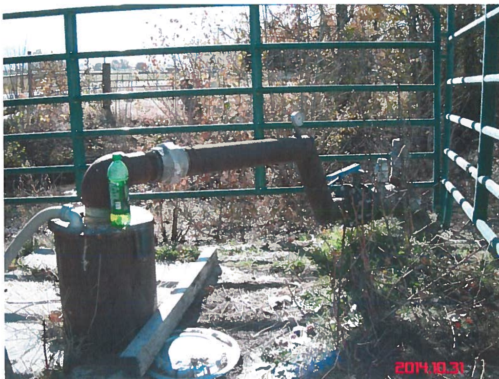
Photo 1: Permit 15-7079 Existing well & primary water supply piping to underground mainline
