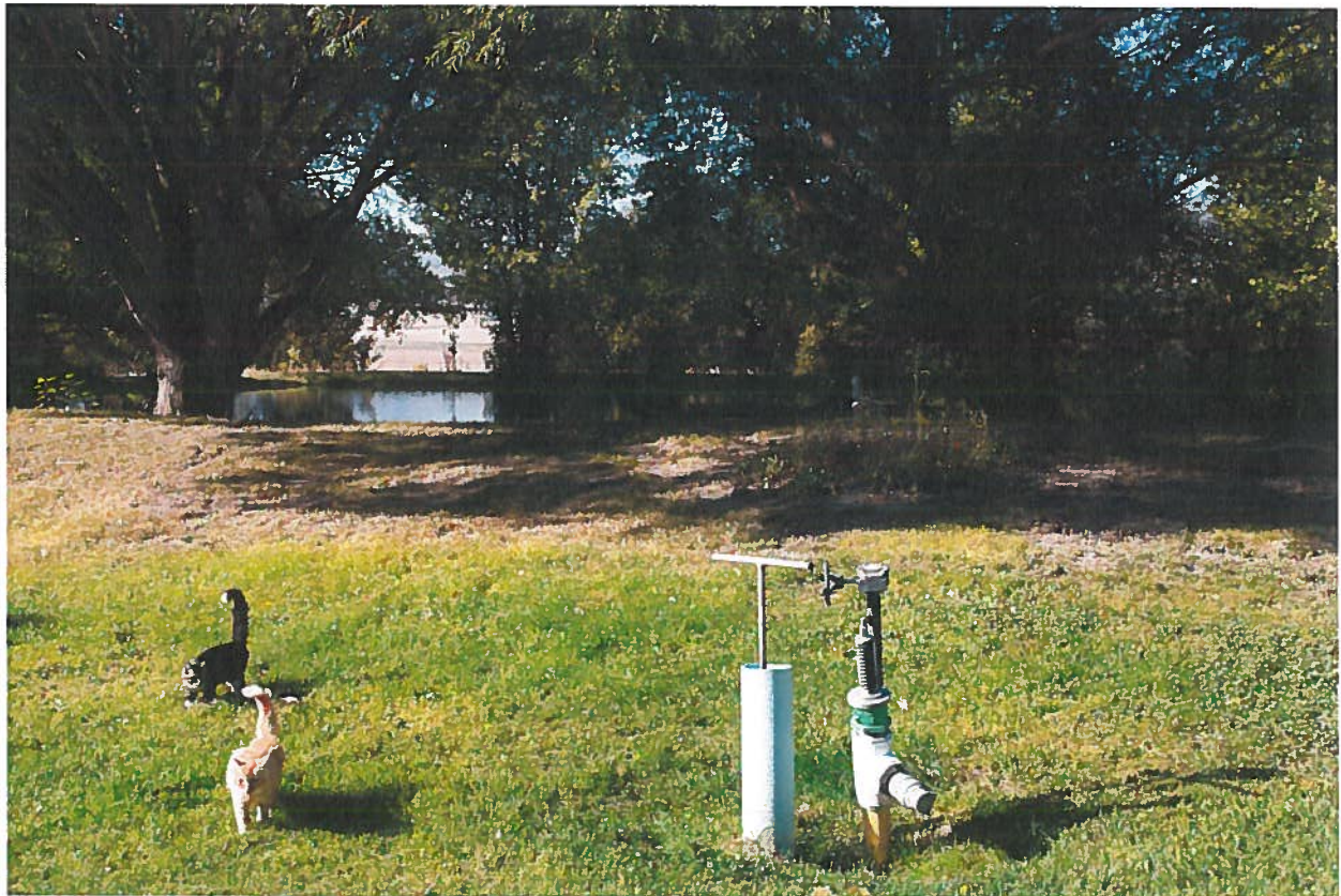
Valve to Pond 1
