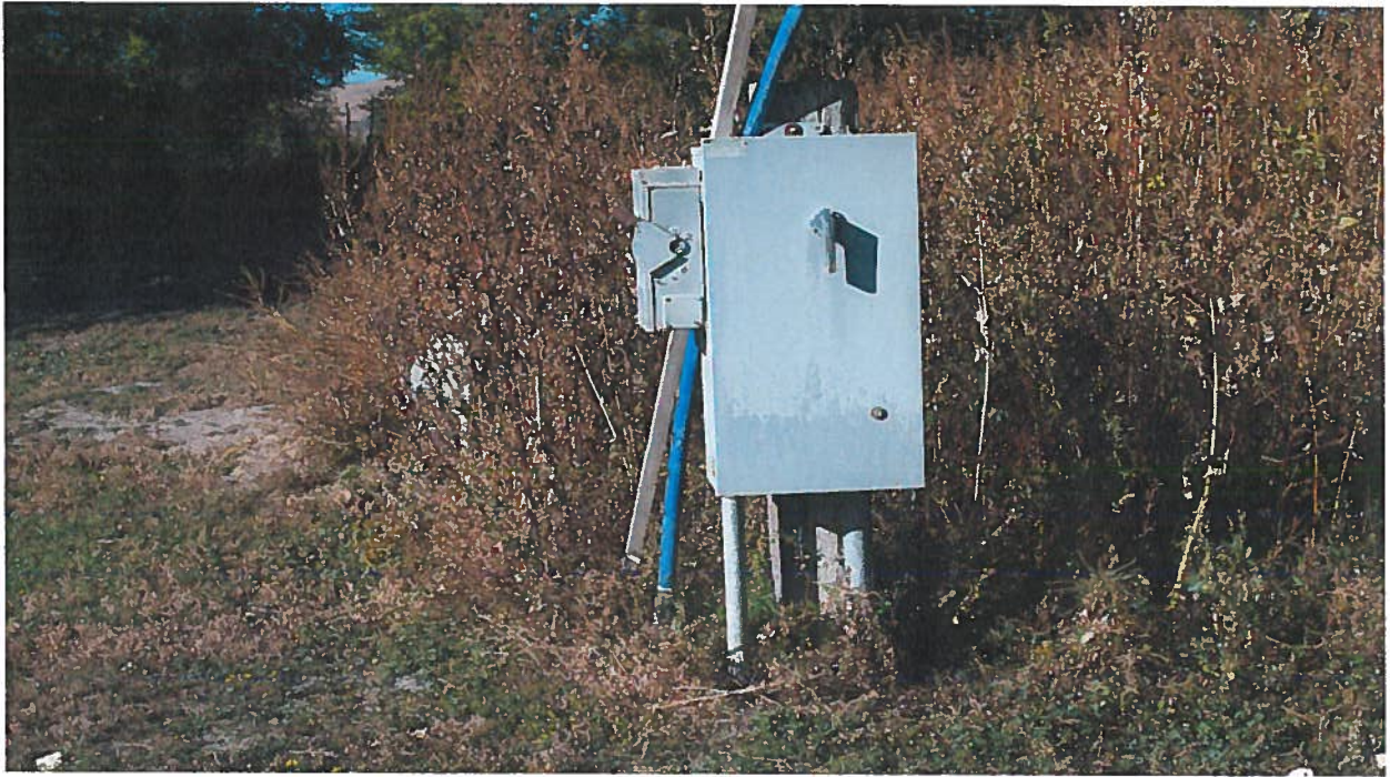
Power Box and Well
