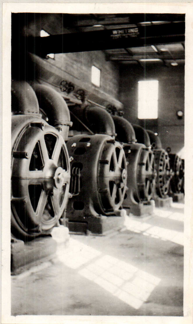
Interior of Pumping Plant No. 1.
