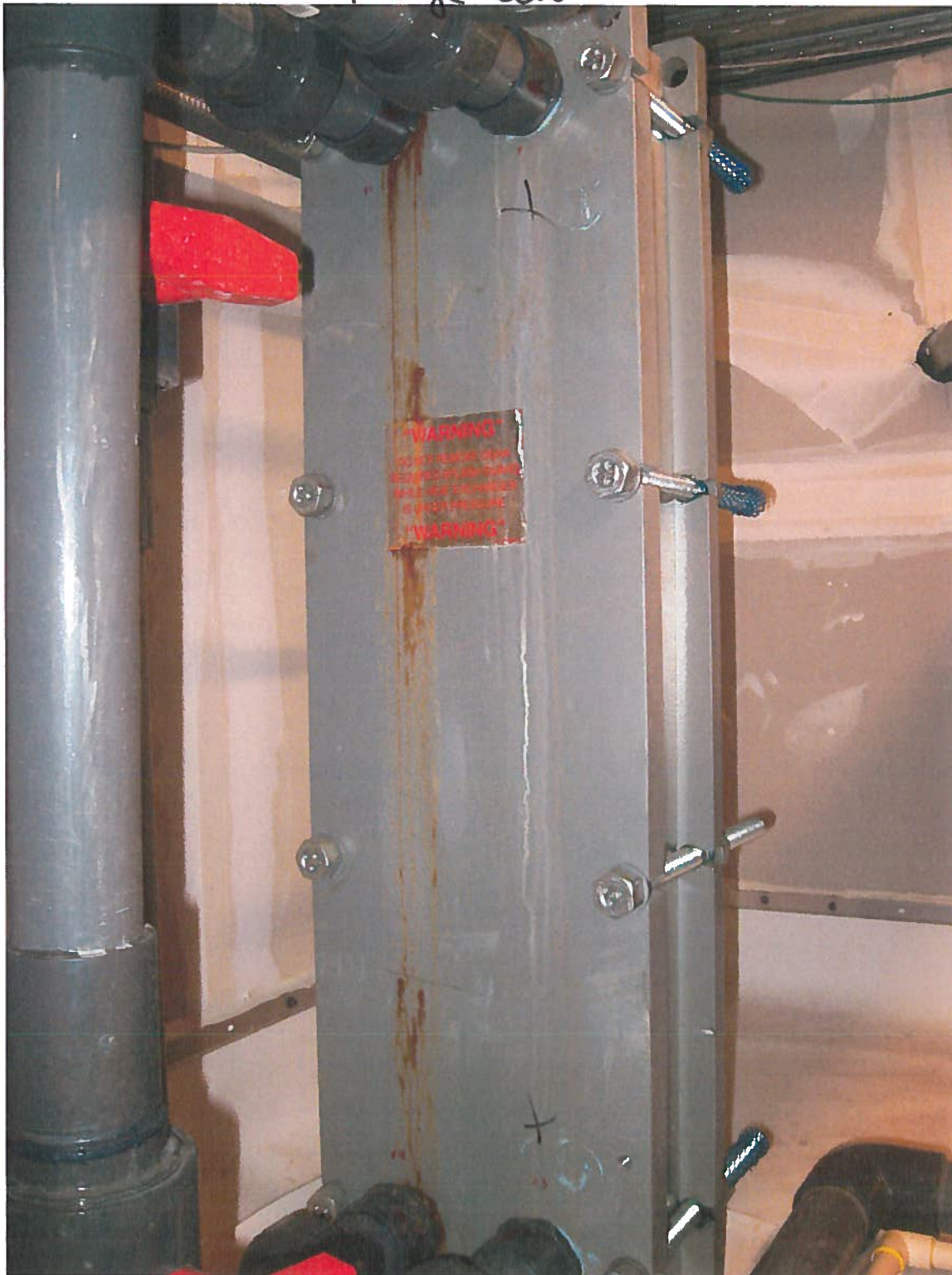
Heat Exchange unit
