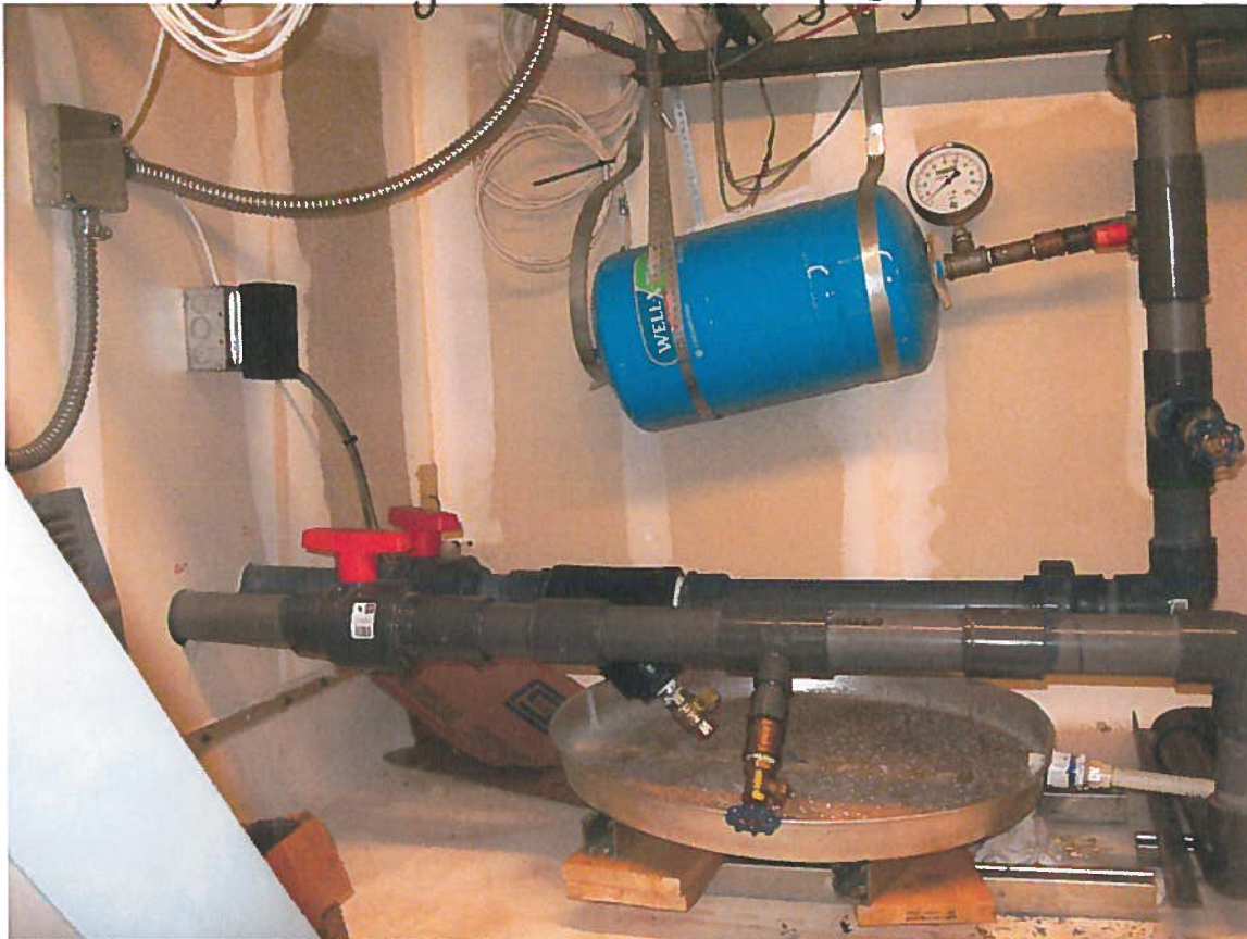
Heating; Cooling water delivery system
