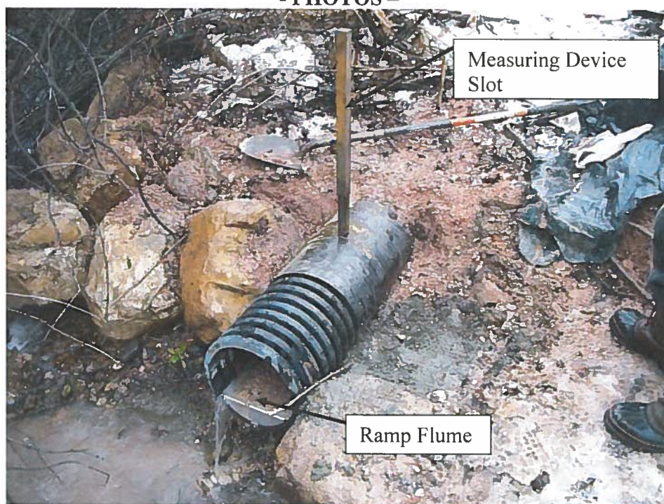
Photo 1 – Bypass Pipe with Flume and Flow Measuring Device Slot
