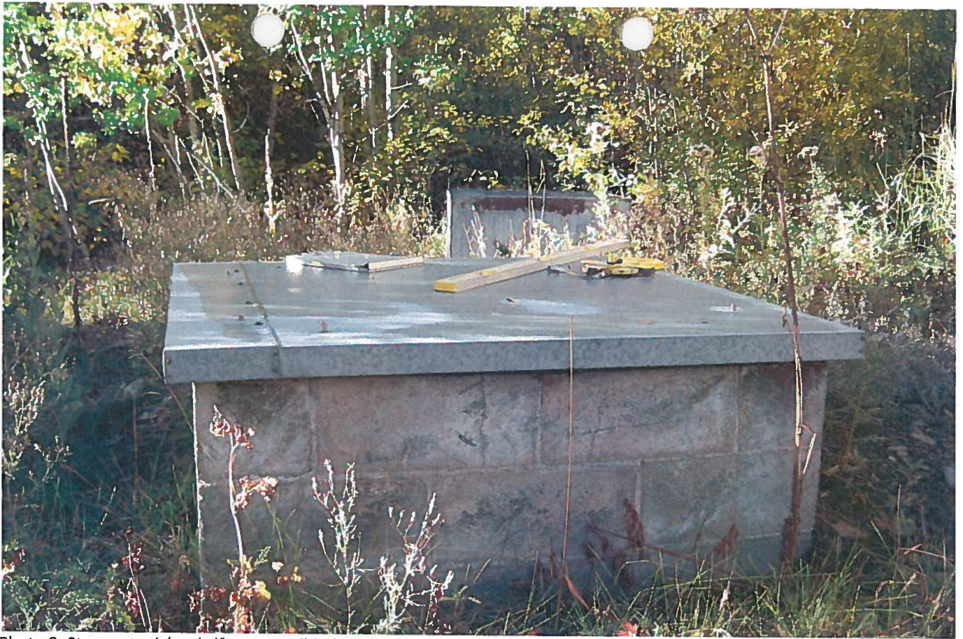
Photo 3: Storage tank/vault (foreground) below weir box (in background).
