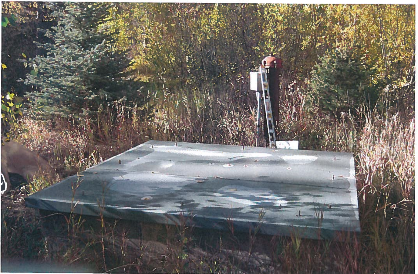
Photo 4: Control structure on edge of property & downstream of weir box & storage tank. Note vertical steel pipe casing behind box with electrical connection for submersible irrigation pump (pump size unknown/could not be confirmed).
