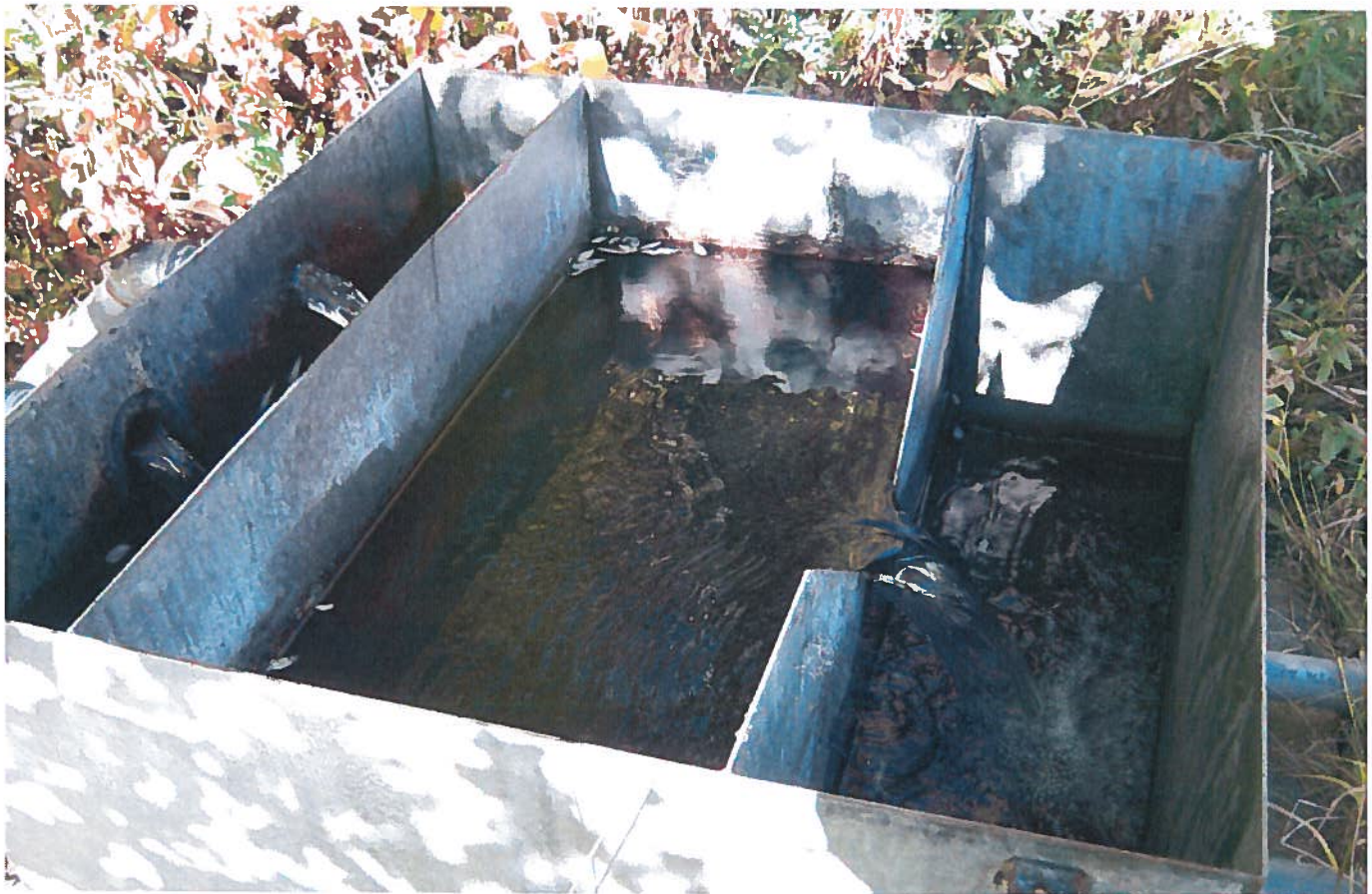
Photo 2: Weir box with two 2 inch pipes inflow from spring source/diversion (left side of photo), and two 2 inch pipes discharge to storage tank (right side of photo).
