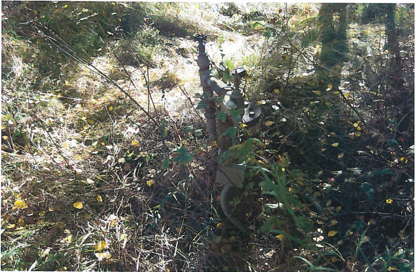
Photo 6: Irrigation well by pond – water right 37-20809 (GPS tag A0017385).
