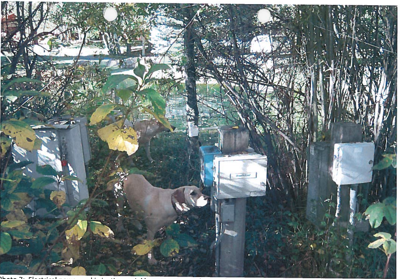
Photo 7: Electrical power and irrigation sprinkler system control panels/boxes (photo taken from irrigation well, pond in background).
