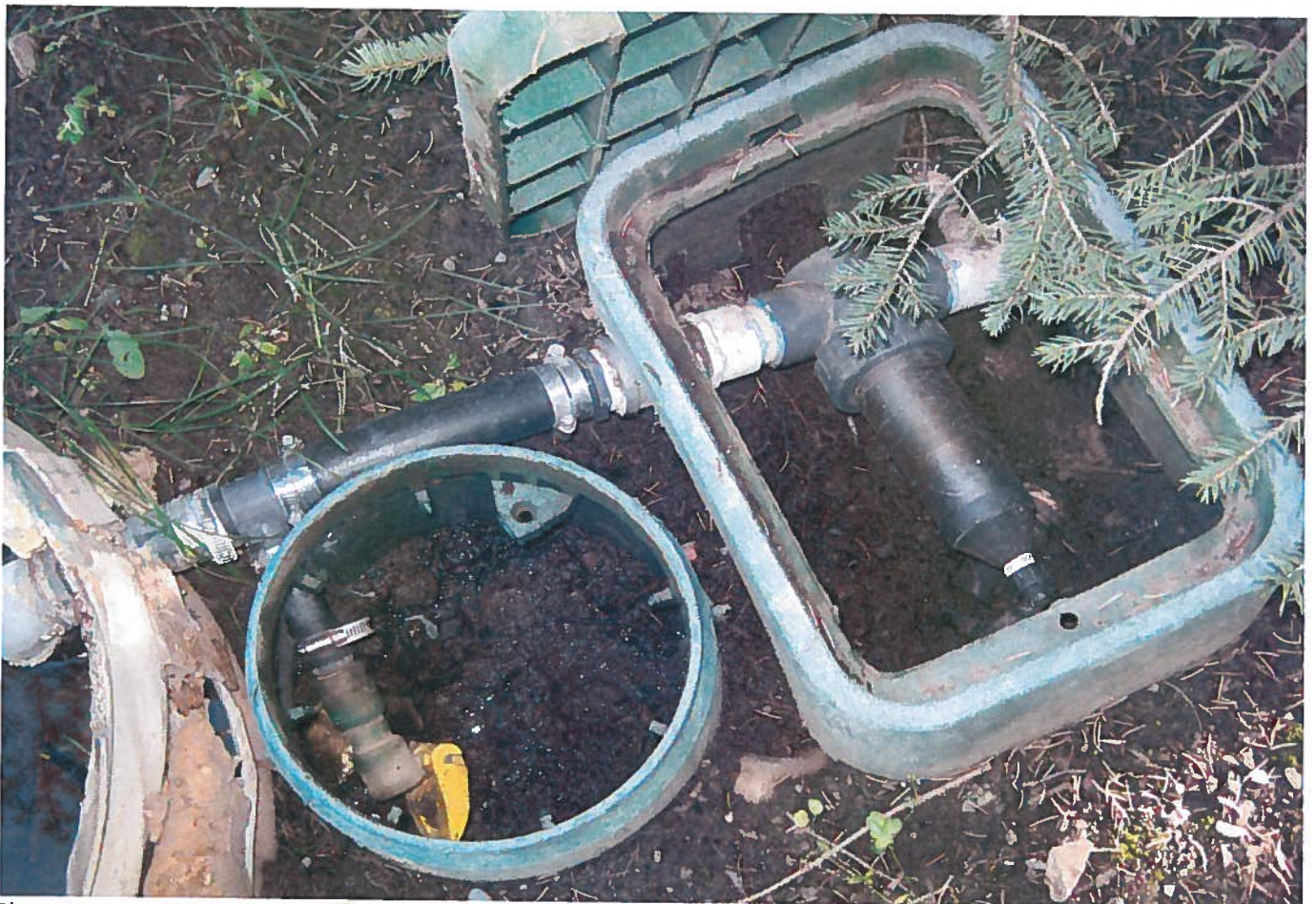
Photo 10: Irrigation box next to CMP/pump with filter/irrigation system connection.
