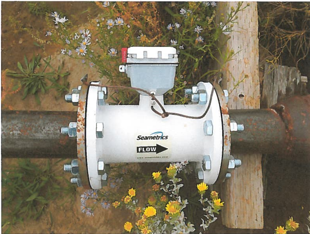
Seametrics meter installed on well
