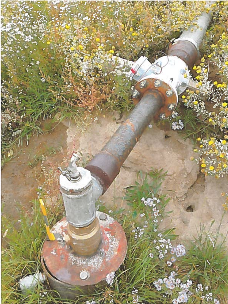
Well and flow meter
