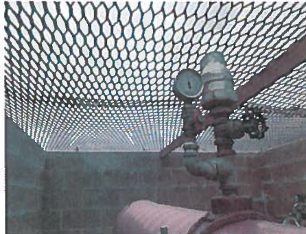
Upper Left & Right: The diversion system at the Columbia Village tap #1 from the main transport pipeline.
