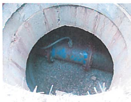
Lower Left & Right: Manhole access to the flow meter at the Columbia Village tap #1.
