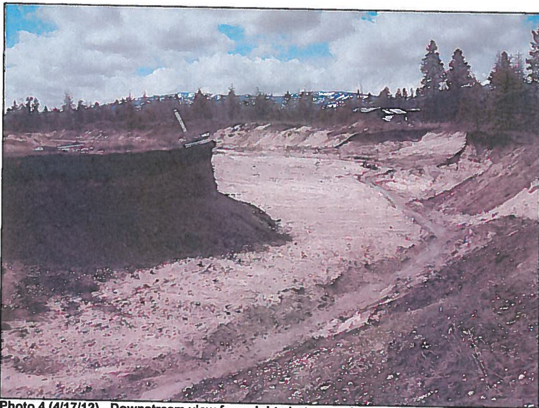
Photo 4 (4/17/12) - Downstream view from right abutment of temporary berm. Note the thick accumulation of sediment that reportedly was washed from the dam failure.
