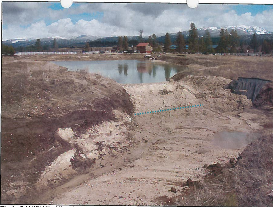
Photo 2 (4/17/12) - View looking upstream at the temporary 7-8' tall barrier constructed ~100 feet upstream from the failed dam location. Note the saturated zone (dashed line) and leaking water near the base of the sand embankment.
