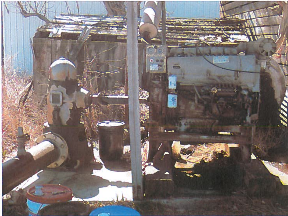
Figure 1: Deutz diesel motor and wellhead.
