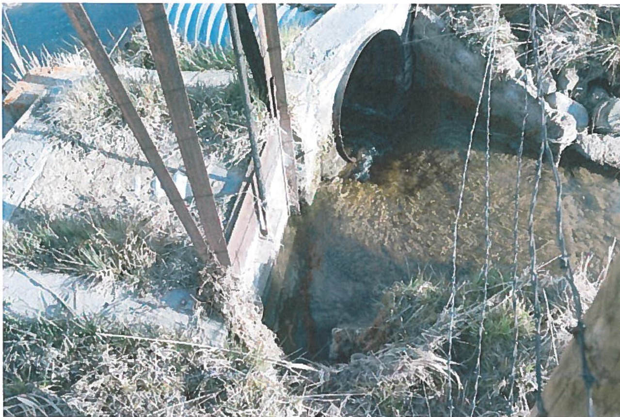
This photo shows the culvert which runs under US 93 conveying water to all permit holders in the Lovers Lane, Wagon Wheel Road area, showing the lockable diversion and potential for measuring flow:
