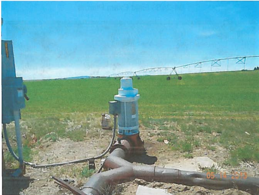
Photo 3 – Well #2 looking south
