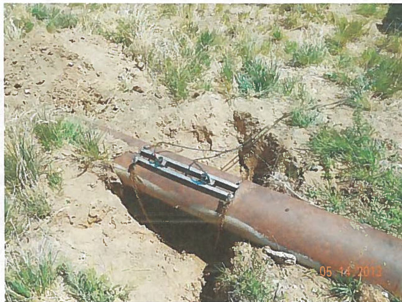
Photo 1 – Transducers installed on pipeline
