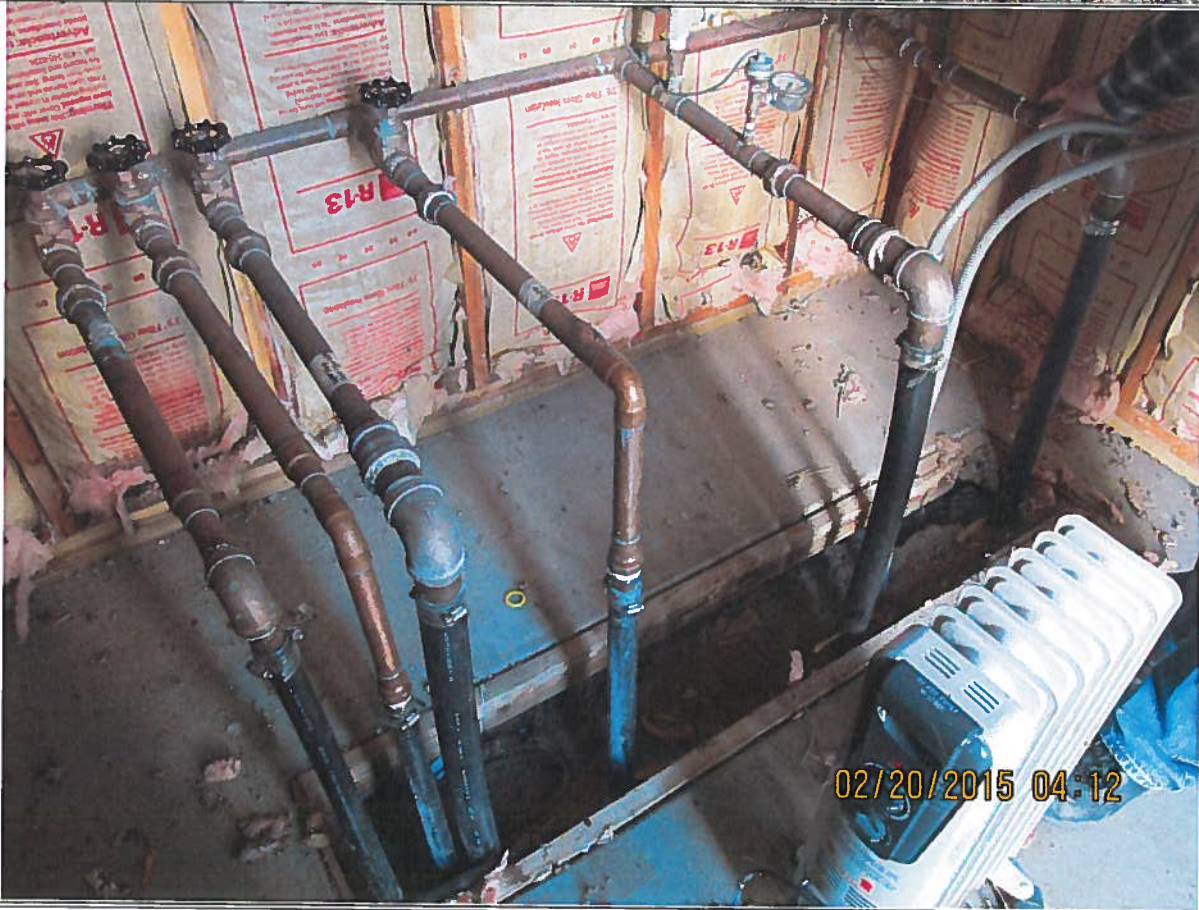
Inside well house. Water lines supply domestic and pond storage use.
