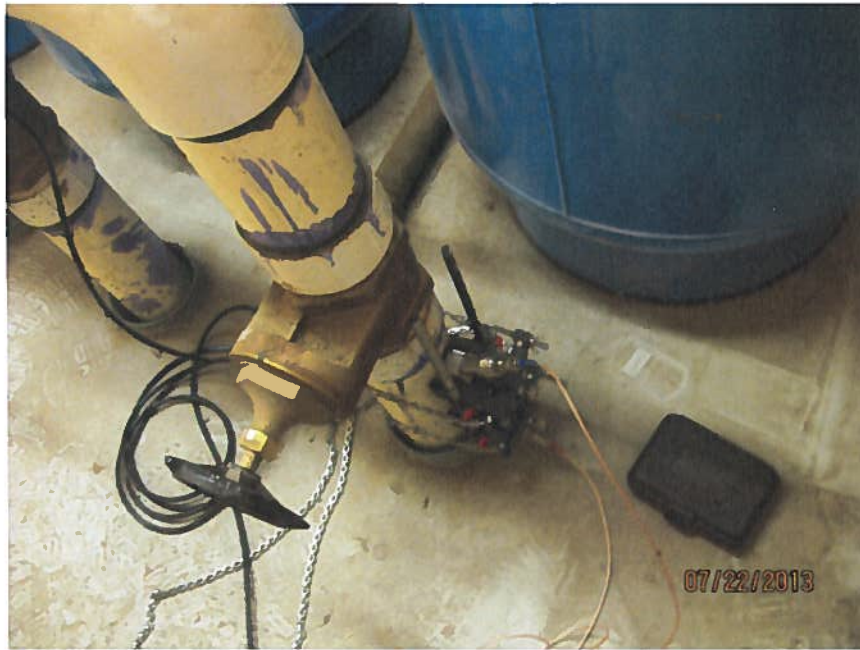
Figure 15: Well #7 measurement location (flow in from well).
