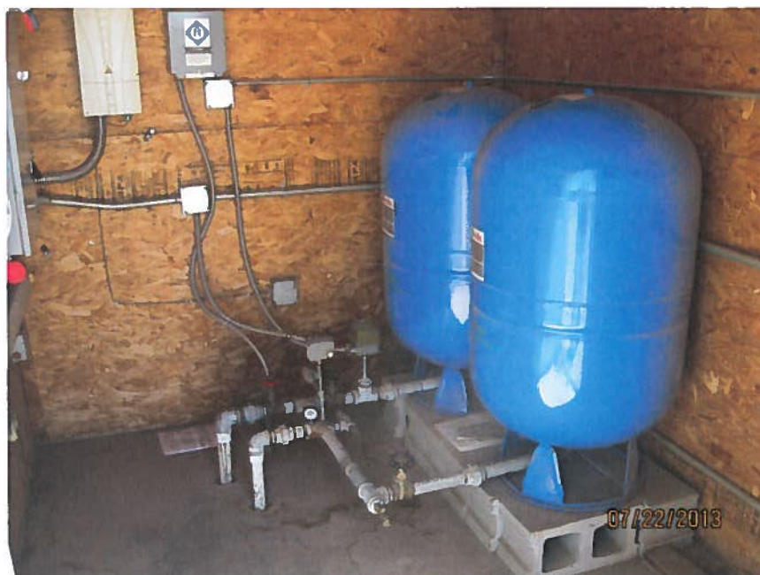
Figure 4: Well #2 pump house plumbing.
