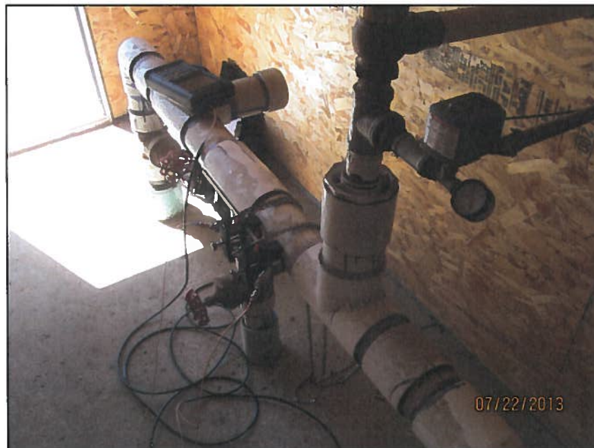
Figure 12: Well #6 pump house plumbing.
