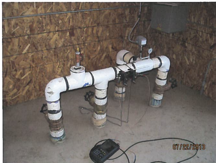
Figure 8. Well #4 pump house plumbing. Valves were adjusted to measure all flow.
