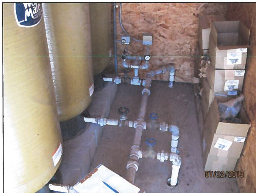
Figure 10: Well #5 pump house plumbing.
