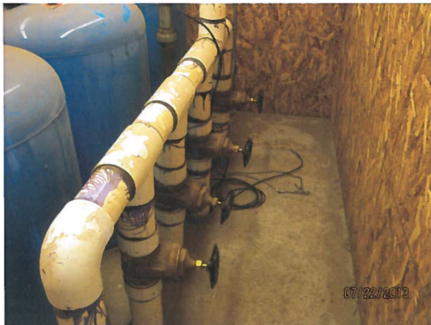
Figure 14: Well #7 pump house plumbing.
