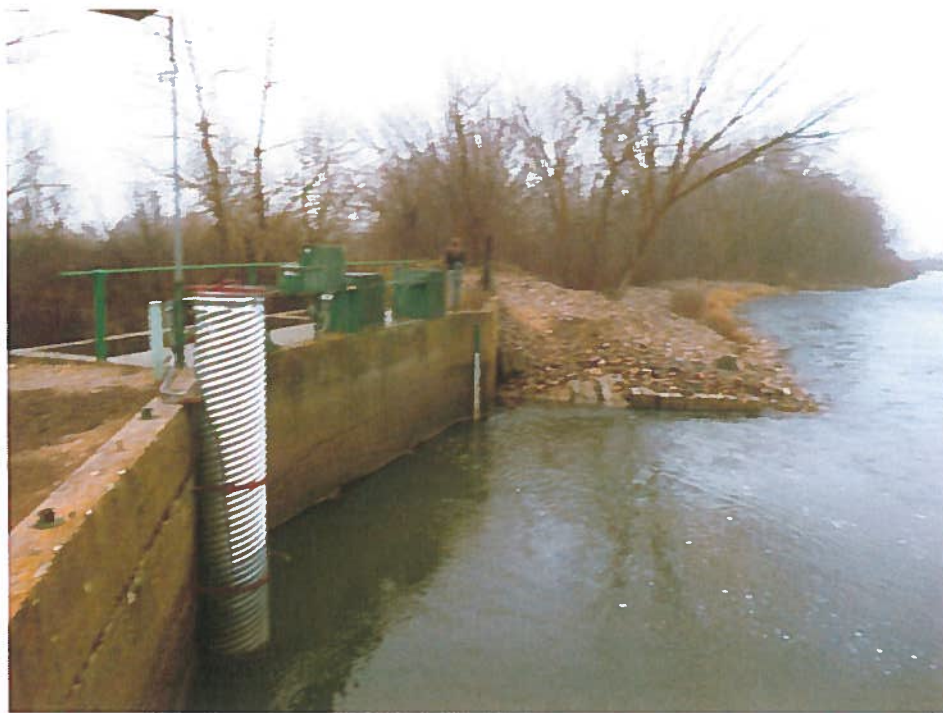
(65-22931, 2/3/15) Gauge station and stationary water depth measurer at point of diversion (43° 52' 11.4600", -116° 34' 12.7200".) At the confluence of the Payette River and Sevenmile Slough on 02/03/15.
