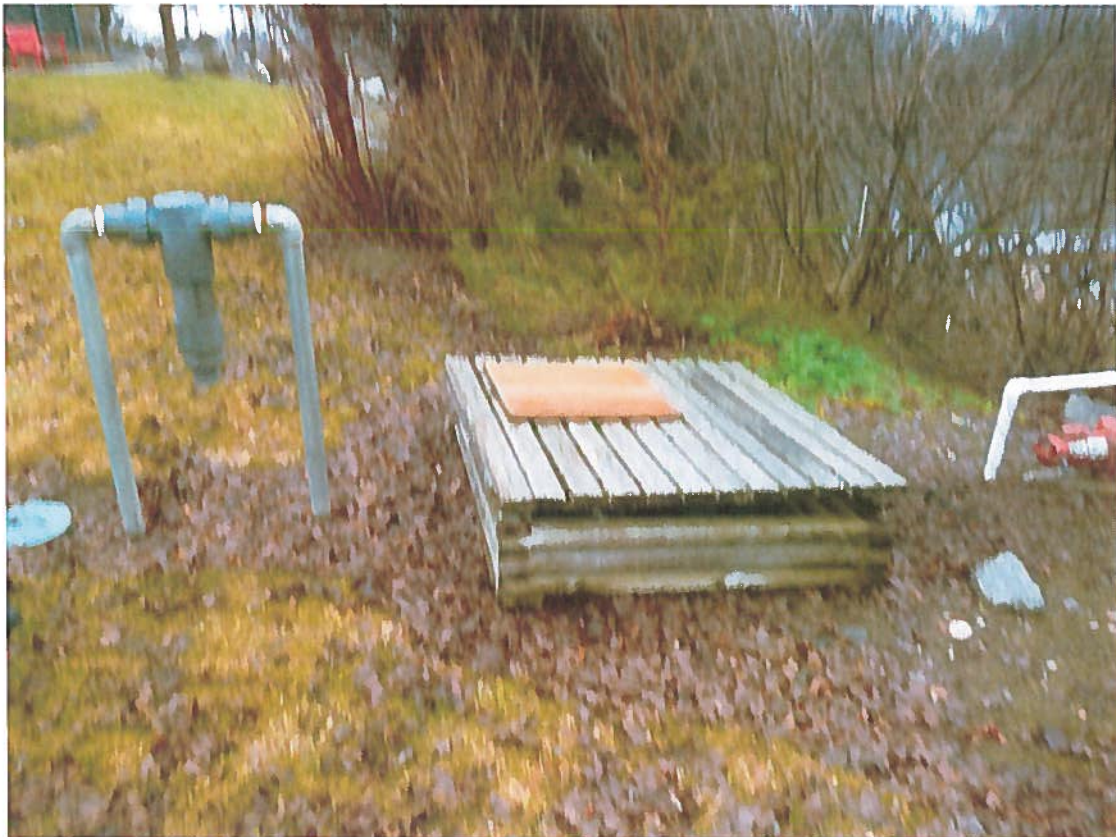
(65-22931, 2/3/15) Wooden vault where motor for point of redirection is located, 15' below surface level, before connecting to sprinkler system. Pump on right side of picture is from older uses and is no longer used. (43° 52' 22.3680", -116° 35' 31.5600".)
