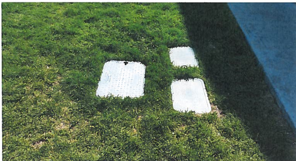
Figure 5: Irrigation sprinkler boxes for common area buried 6-zone sprinkler system.
