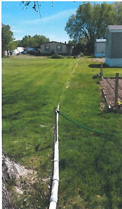
Figure 4: Typical 2-inch above ground PVC mainline running along the backside of the home lots.
