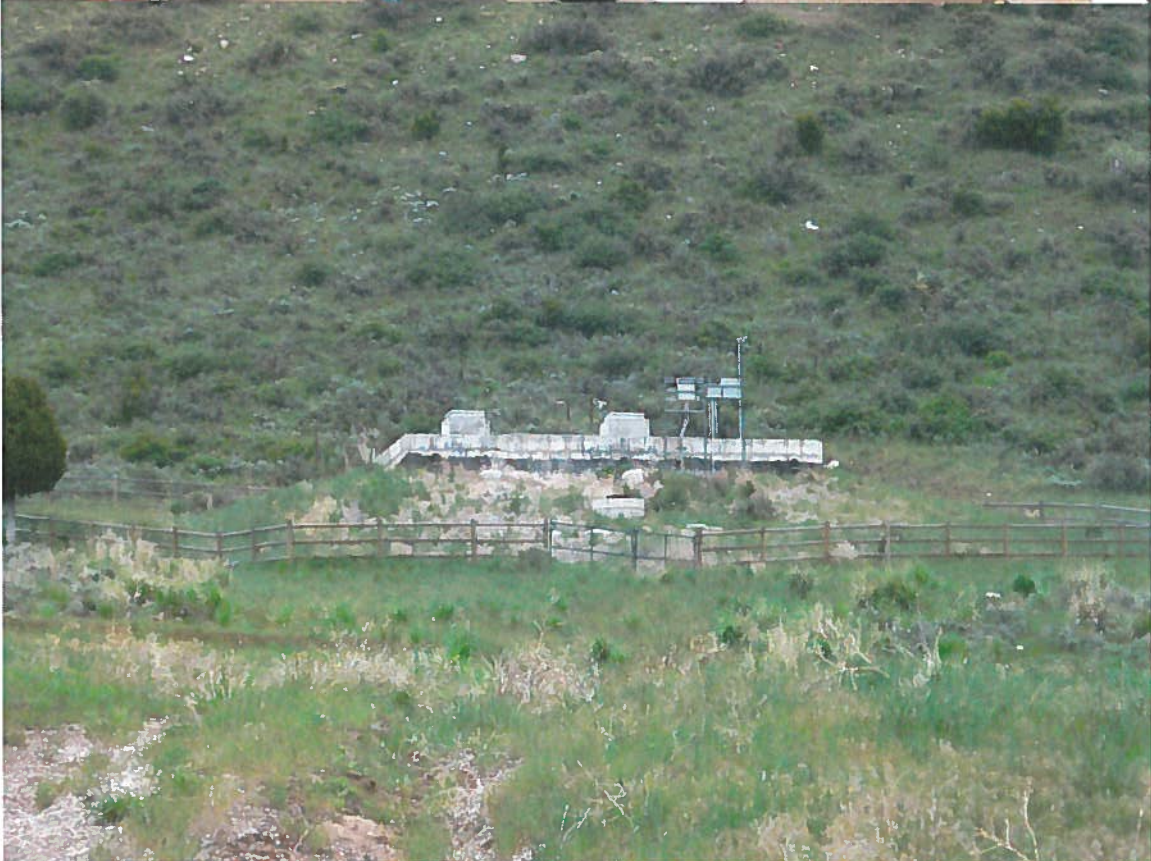
100,000 gallon storage tank
