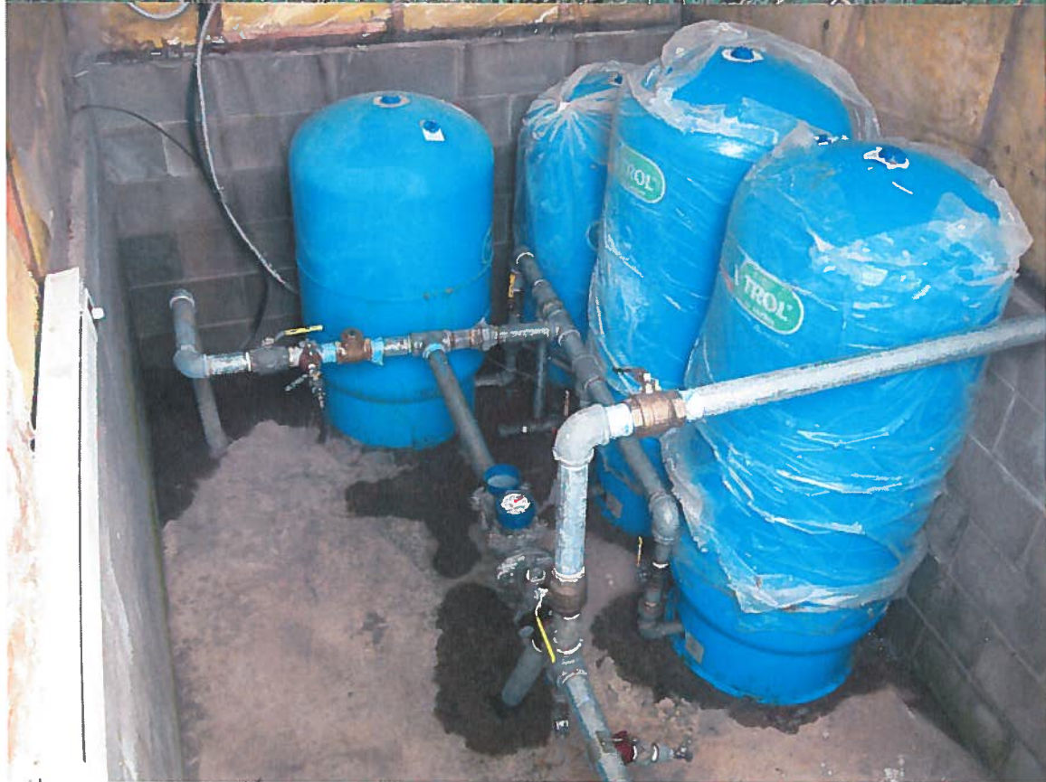
Inside "old well" pump house
