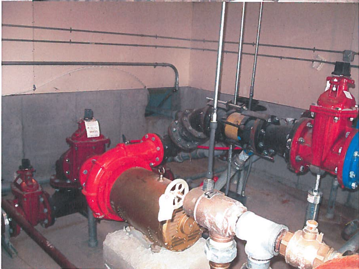
Inside "New well" pump house
