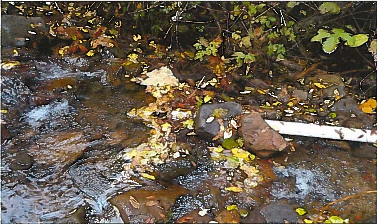
Point of Diversion: View of a screened 3" PVC intake pipe in Trail Creek.
