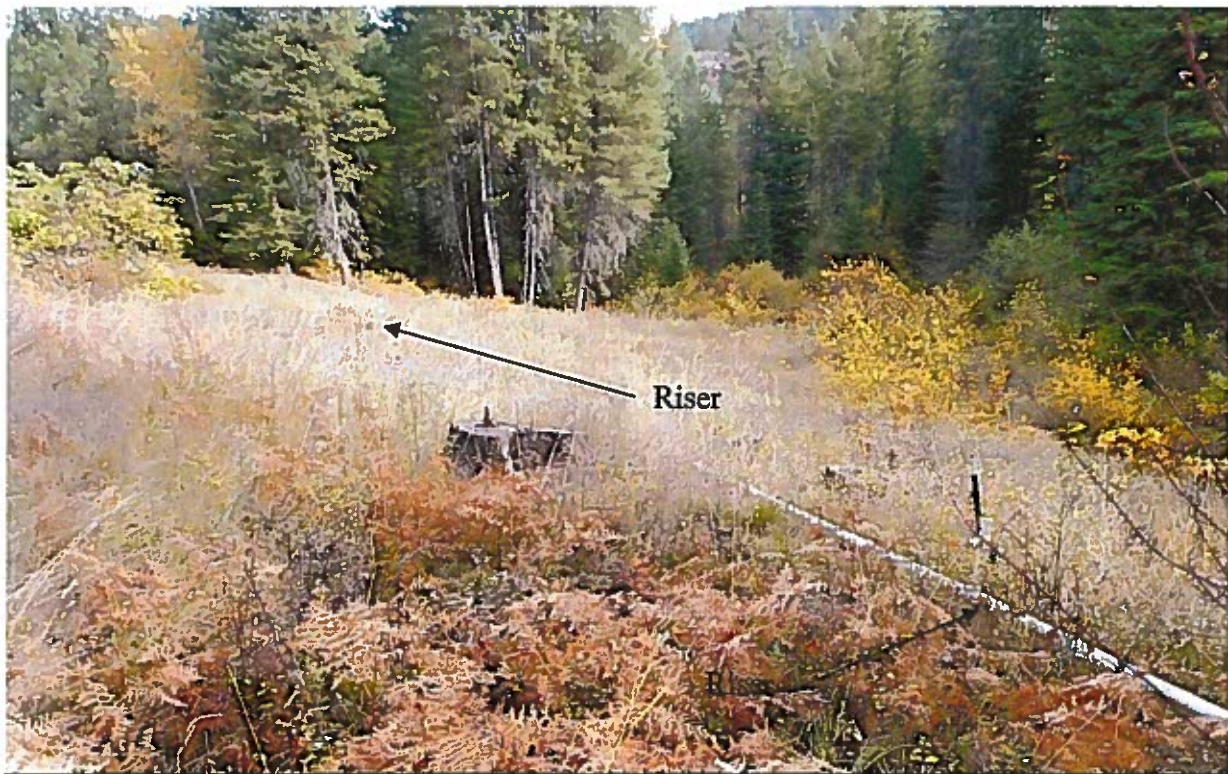
View easterly of the 3" PVC supply line located near the southerly boundary of the right holder's property. PVC risers are randomly located on the 3" PVC supply line for pipe or hose attachment.
