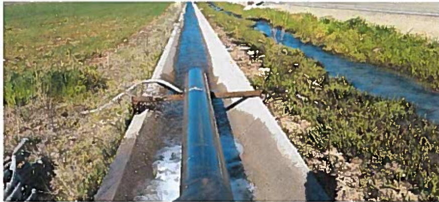
Figure 2: Looking west at the north gravity ditch. Discharge from the NENW well's 8-inch pipe into a 3 foot width x 1.5 foot deep concrete trapezoidal gravity ditch at the north end of the property running westerly along the south side of Lake Hazel Road.
