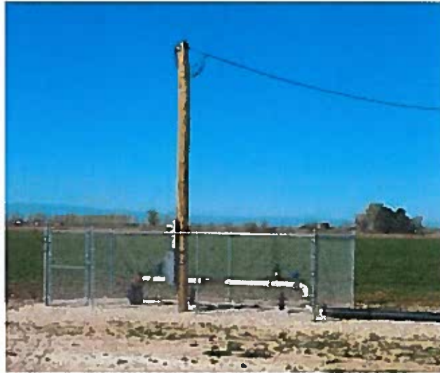
Figure 1: NENW well facing westerly. The NENW well discharges groundwater into a system of 8-inch pipes to deliver water to gravity irrigation ditches at the north end and southern half of the property. The gravity ditches run to the west and water is gravity fed to the fields with siphon tubes.
