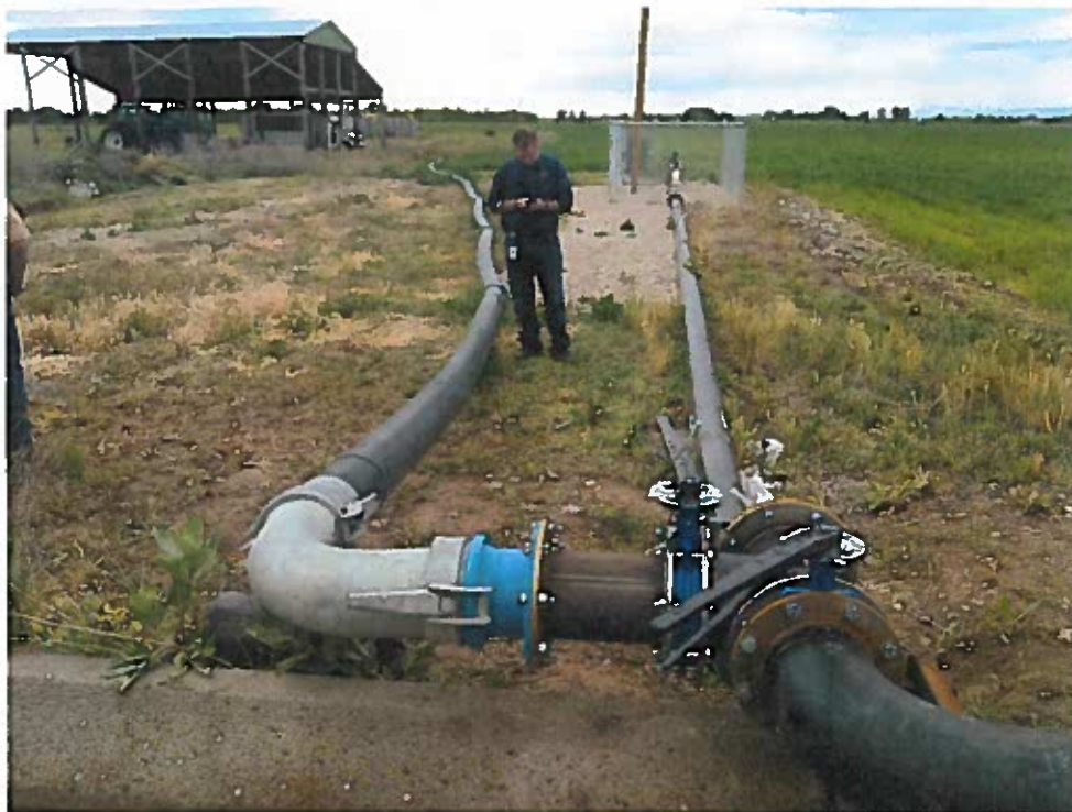
Figure 4: Looking south from the north edge of the property at the well (in the background) and the manifold valves that are used to direct water to the north gravity ditch (right branch in photo) and/or the south gravity ditch (left branch in photo).
