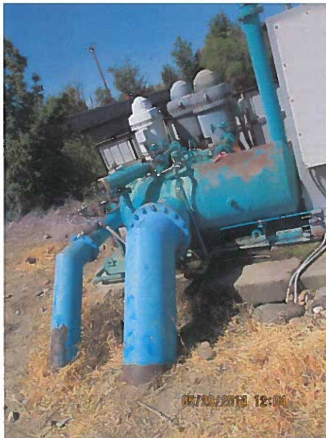
Elbows in discharge pipes caused turbulence making it impossible to get a good measurement.
