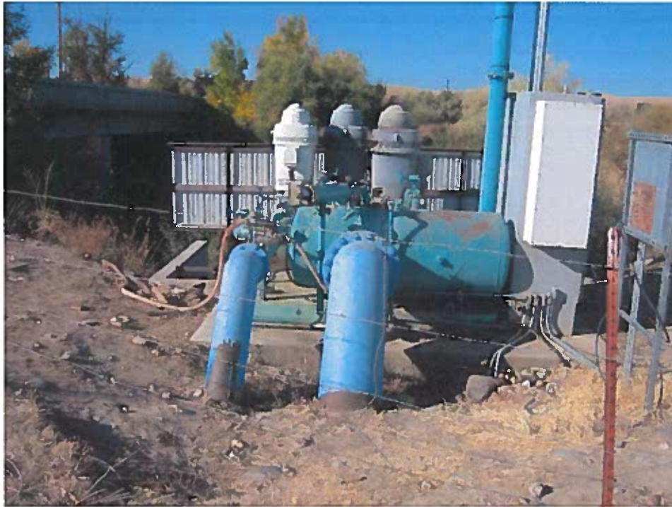
Pumping station from Bruneau River – gray pumps 150 hp, white pump 100hp
