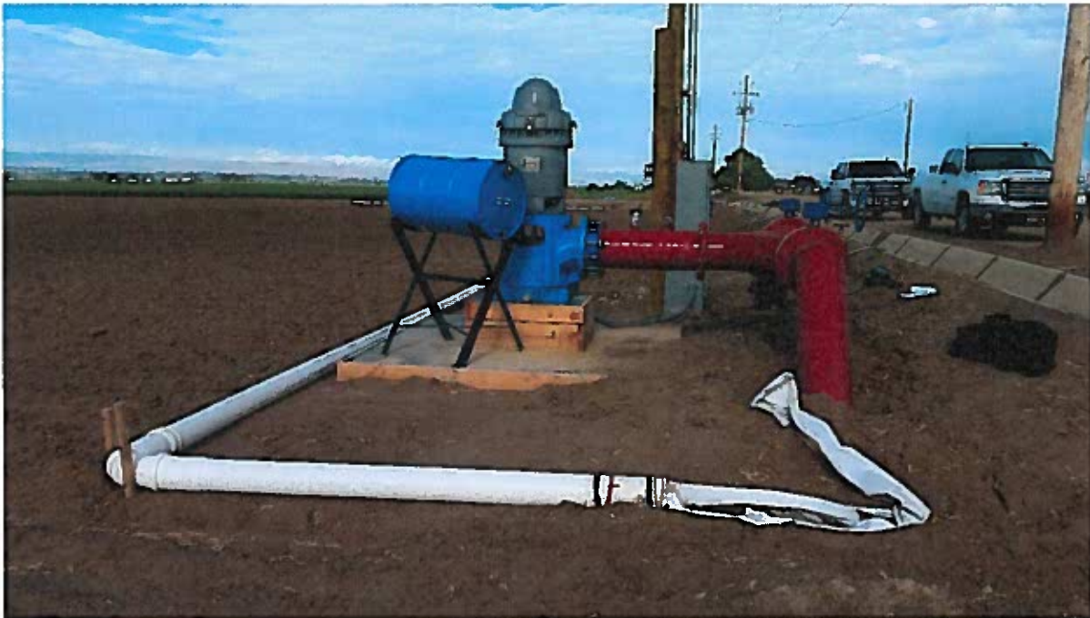
Figure 1: NENE well facing westerly. Ground water from the NENE well is discharged into an above ground 12-inch steel manifold with branches to the east and west. From the manifold, the steel pipe dives into the ground, and 12-inch 100 psi PIP runs underground to the east to one 8-inch open discharge pipe, and to the west to three additional 8-inch open discharge pipes into concrete field ditches.
