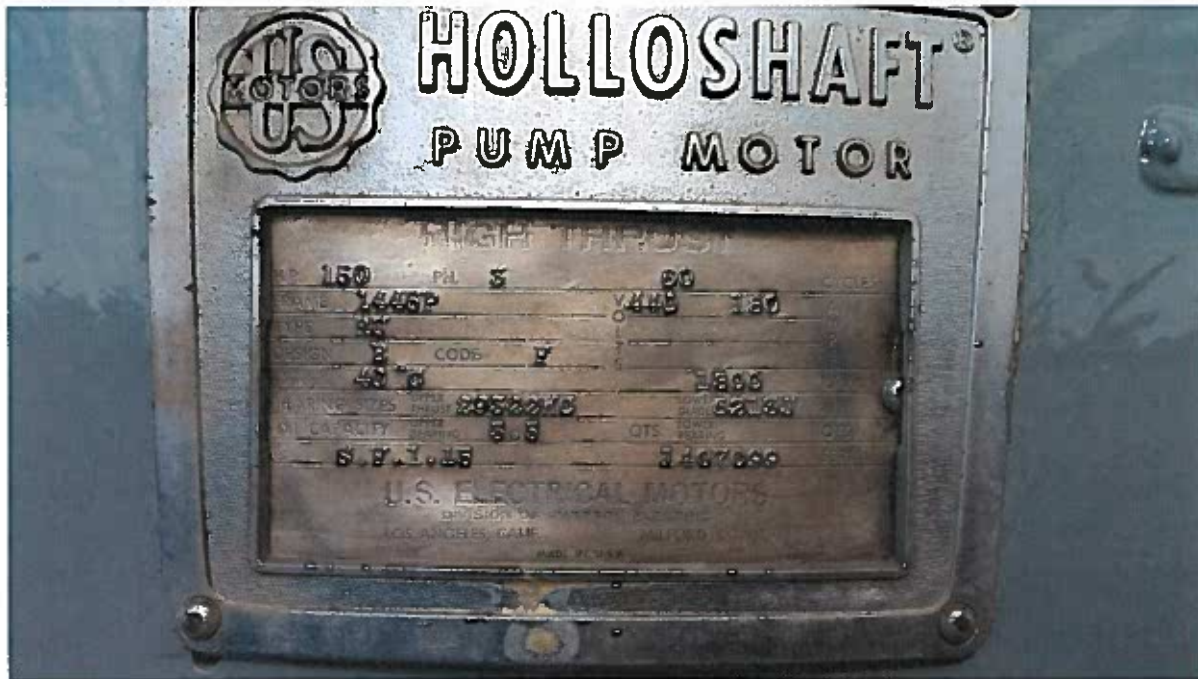
Figure 3: Motor tag showing 150 hp motor installed
