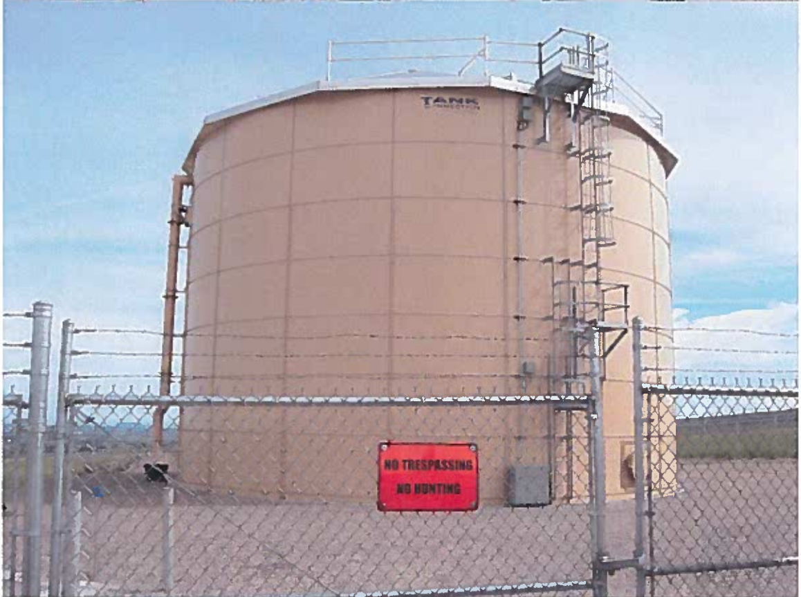
560,000 gallon storage tank
