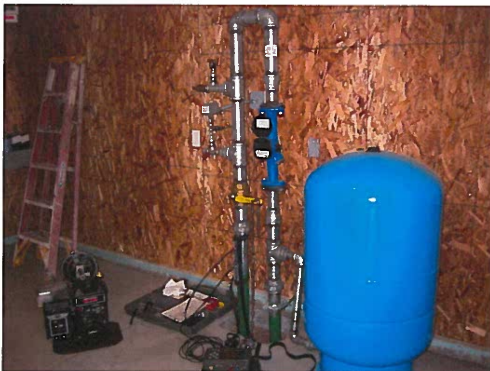
Plumbing Inside Pump House
