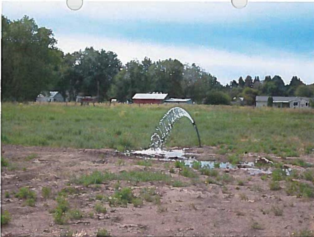
Stub Out With Water Flowing
