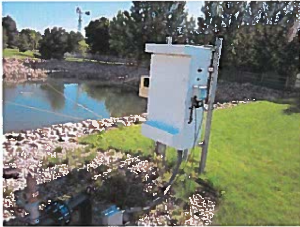
Control Panel for Irrigation System
