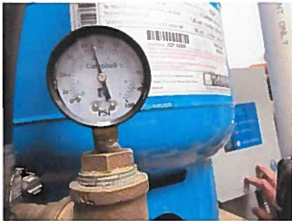
Pressure tank in house
