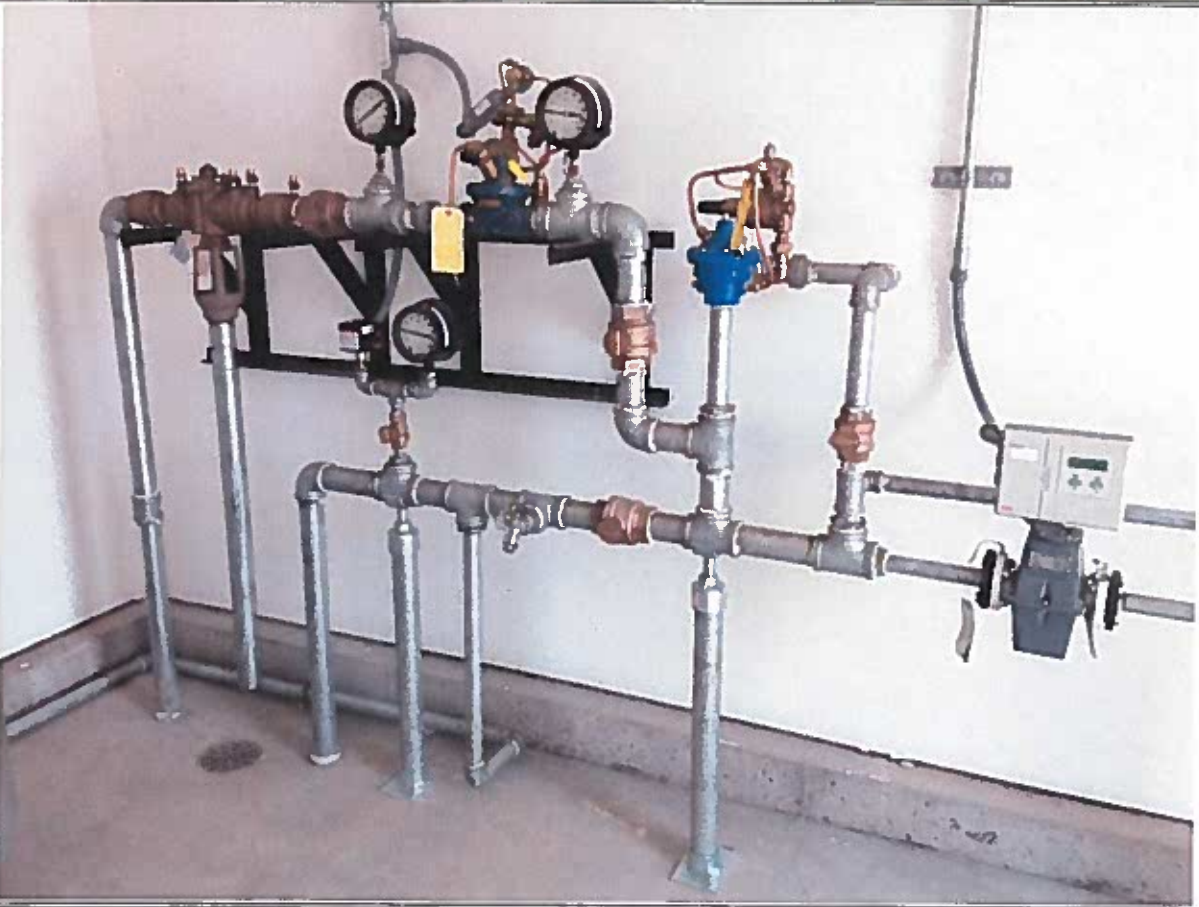
Pump house piping. System has a flow meter (right) that was not operating at the time of the exam.
