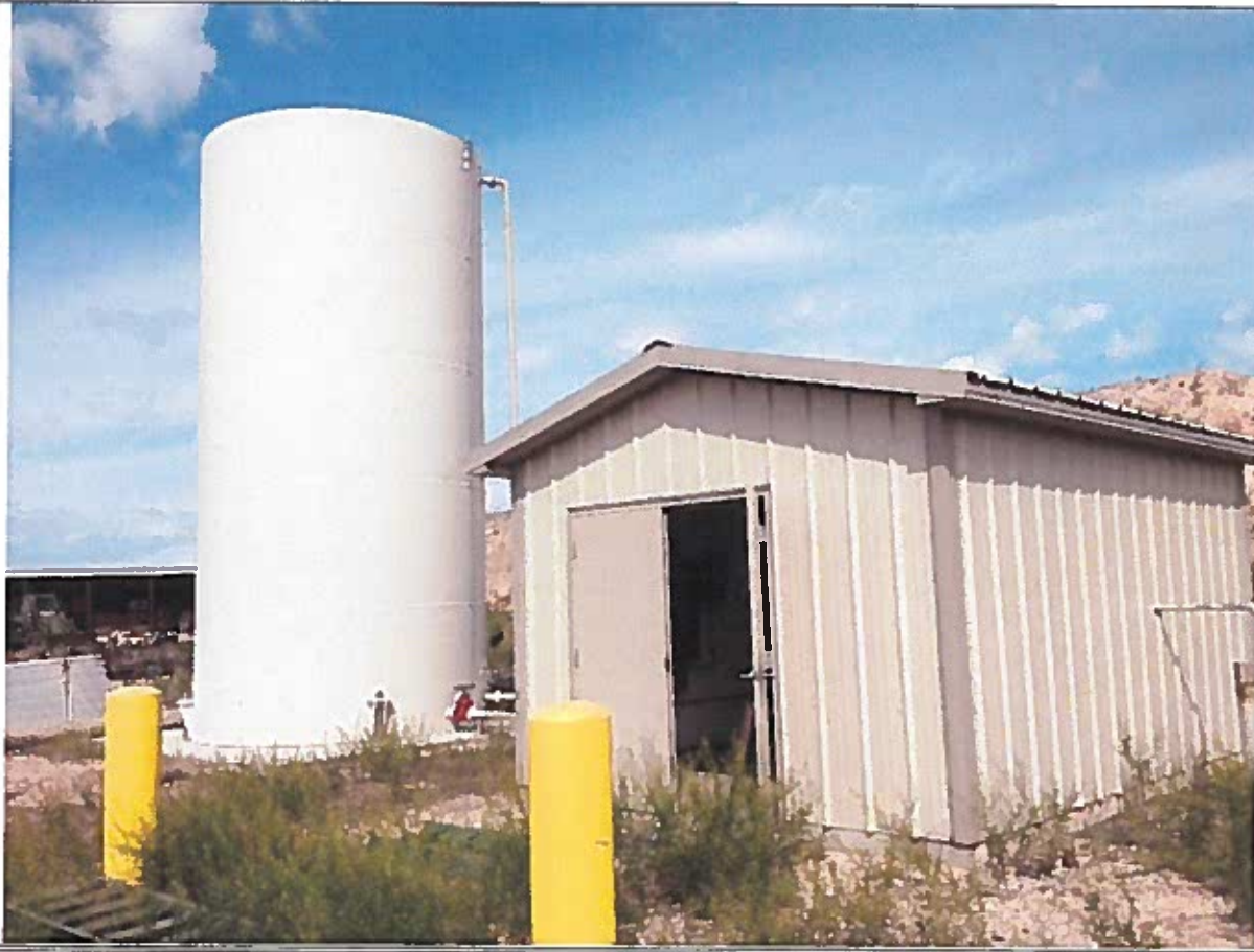
Pump house and 10,000 gallon storage tank
