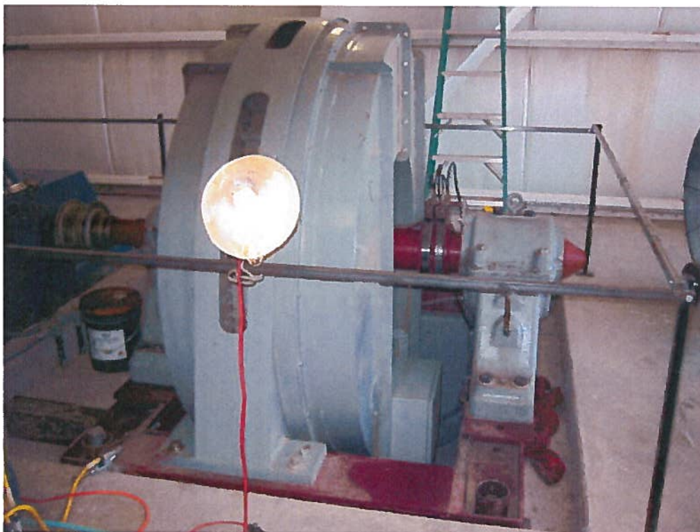
The Westinghouse generator inside the power house
