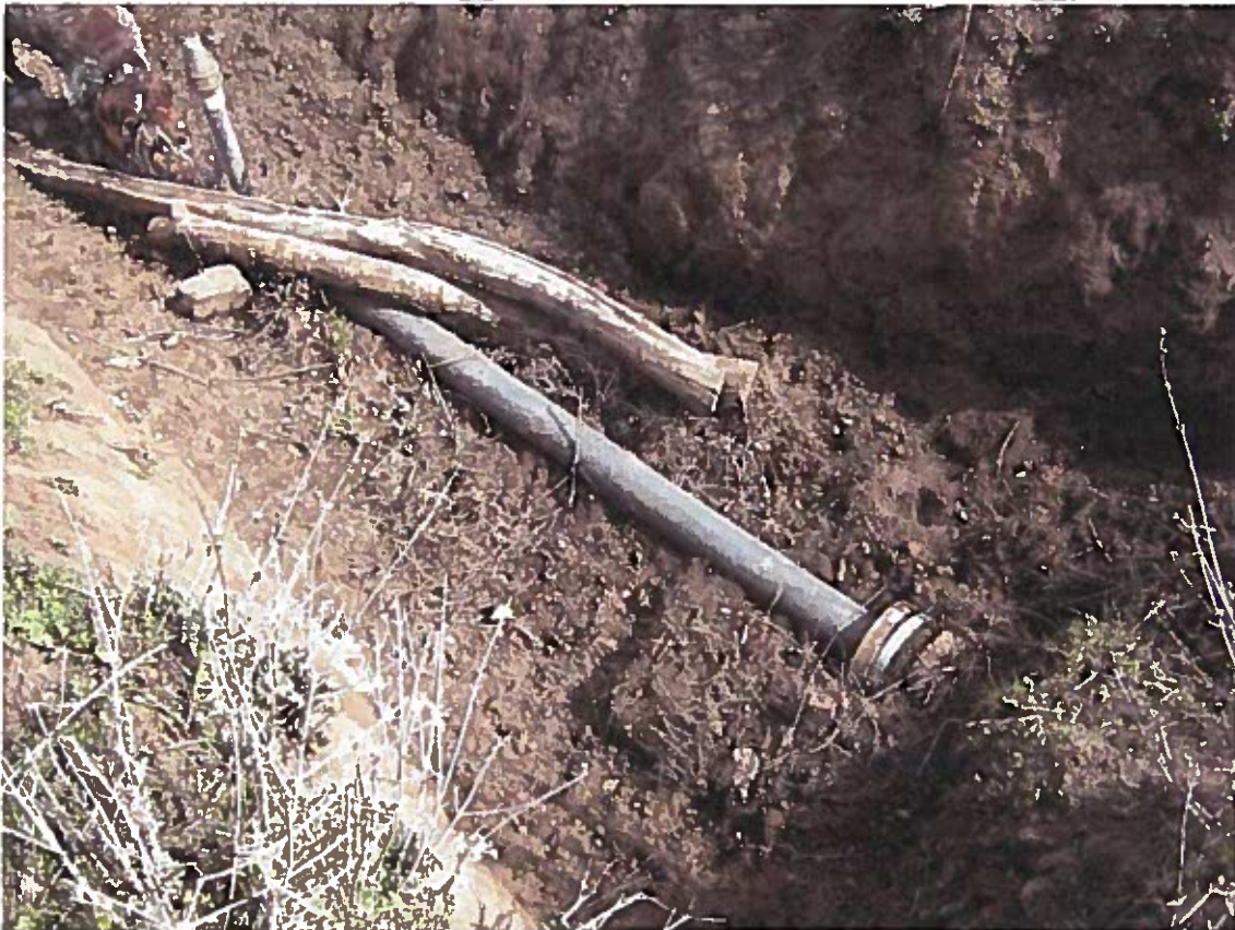
Figure 7 Mullinix 4 inch lateral pipe from mainline (no longer used). Valve with removed control handle on right.
