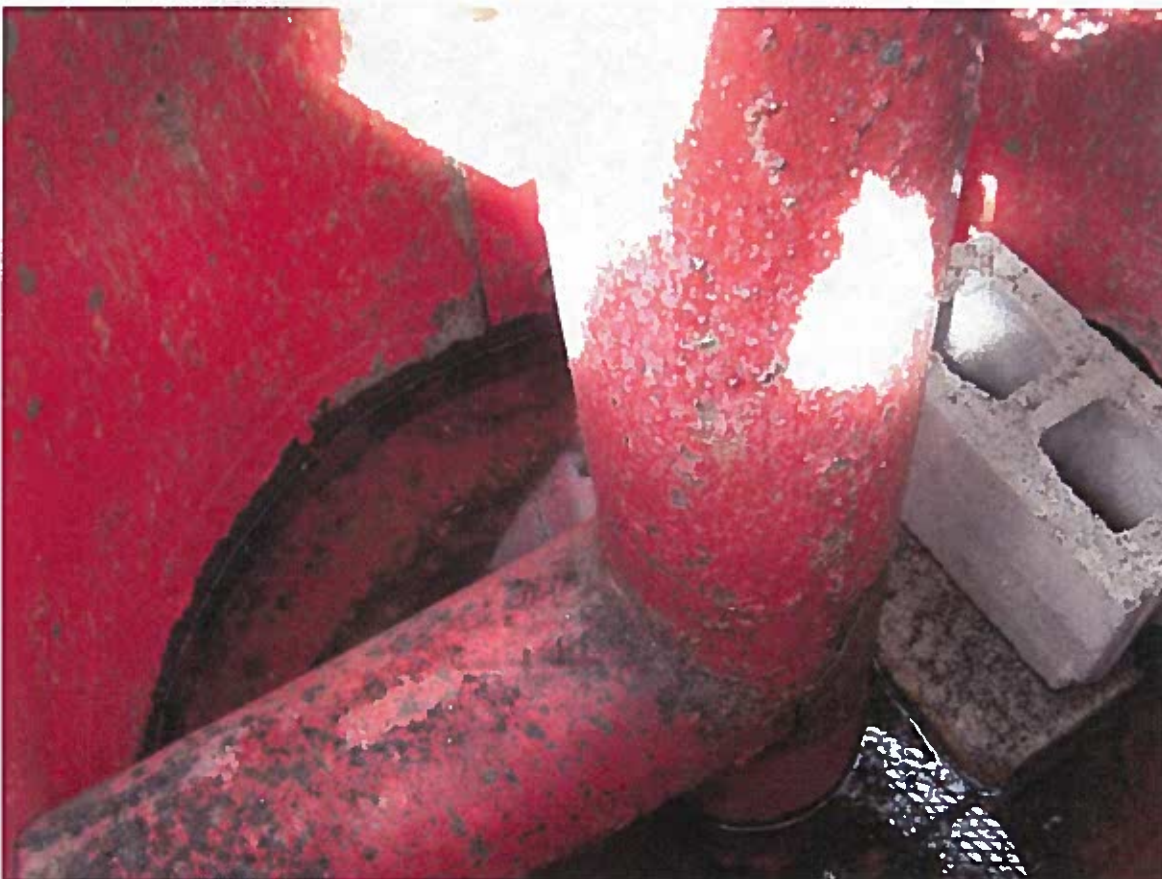
Figure 4 Vertical 8 inch pipe in bubbler canister. Discharge pipe from bubbler on right behind cinder blocks.
