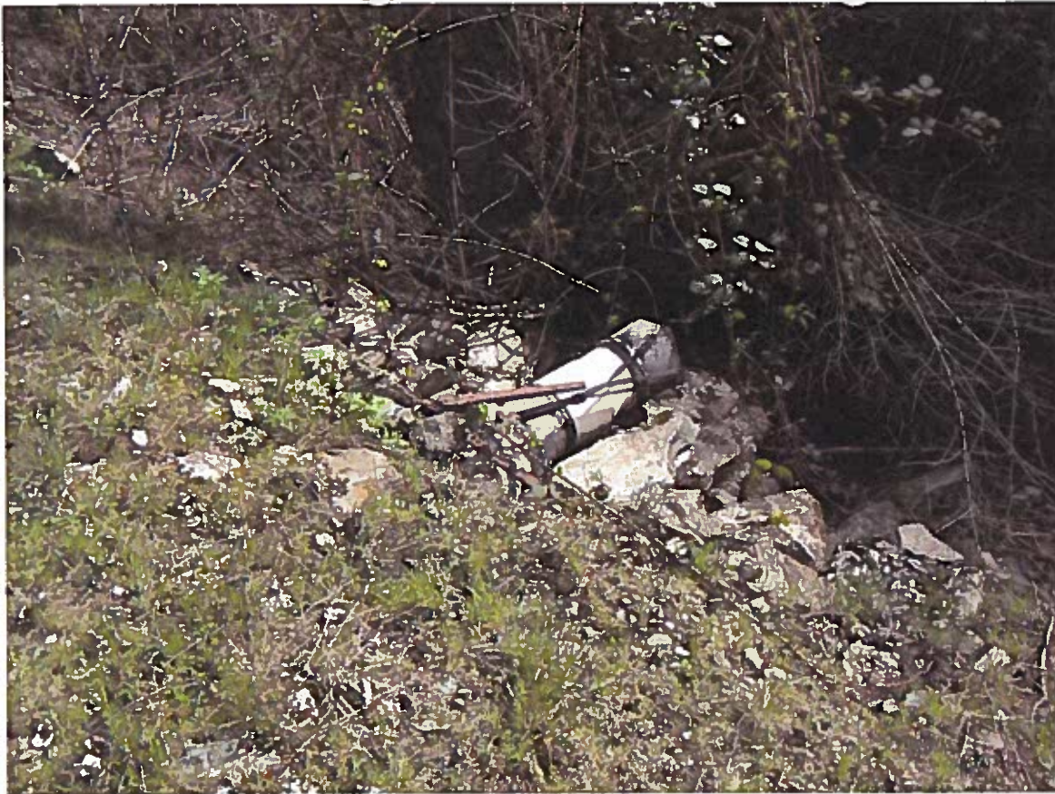
Figure 5 Pressure relieve discharge pipe and valve, discharges or spills water back to creek from mainline below bubbler.
