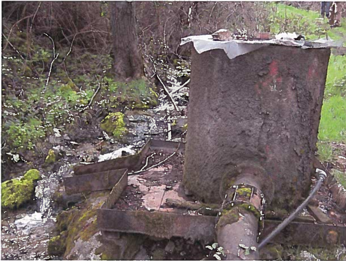
Figure 3 Bubbler on catchment tray with discharge spout to creek. Note 2 inch poly pipe on right to Robinson parcel.
