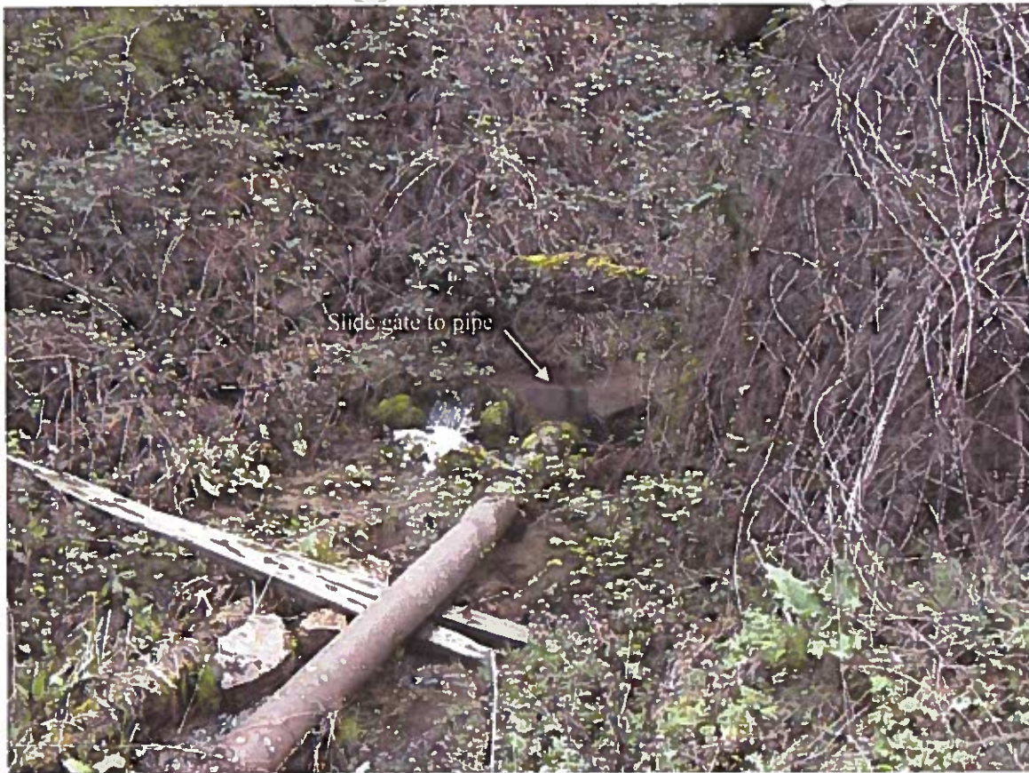
Figure 1 Head gate diversion and 8 inch steel pipe from Joe Creek
